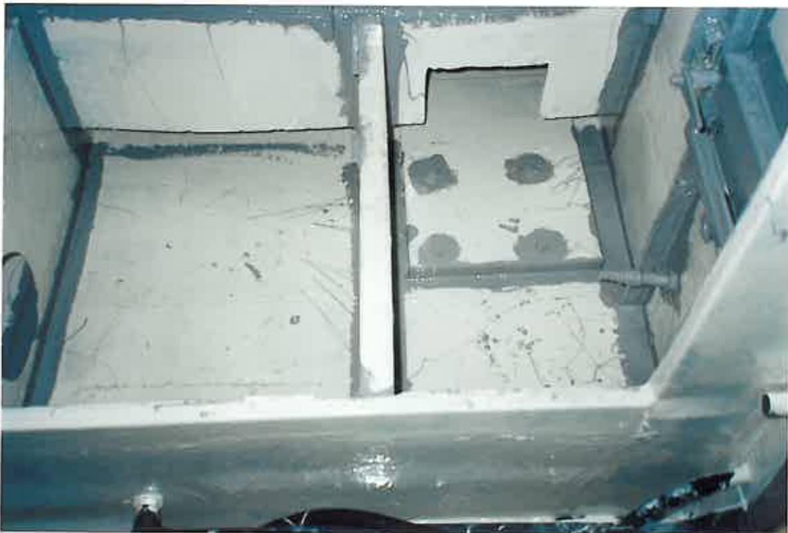
These photographs show the final application of the 2 nd coat of 3M Scotchkote™ 165PW (grey) in order to achieve a total, nominal dry film thickness of 1000 Microns (1mm), and between 1500-2000 Microns (2mm) over all stripe coated areas.
