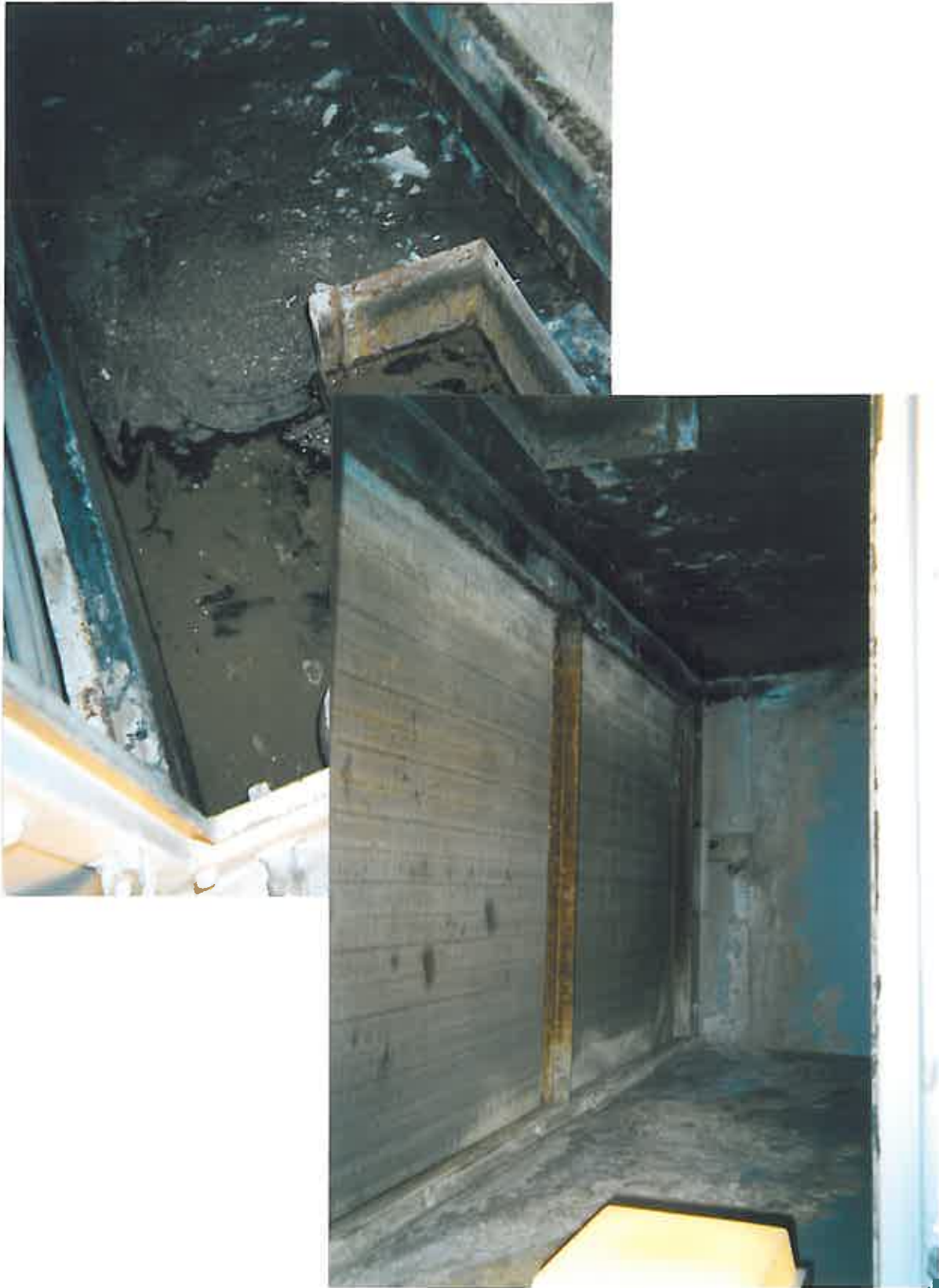
The above photographs show the internal condition of the AHU, prior to any preparation work being carried out. As the photographs clearly show, the existing Bitumen coatings had failed with signs of progressive corrosion, which in areas was applied up to 30mm in thickness.
