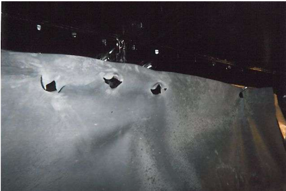
These images show the tank after being drained of water and before / during removal of the failed butyl liner, felt lining and insulation.
