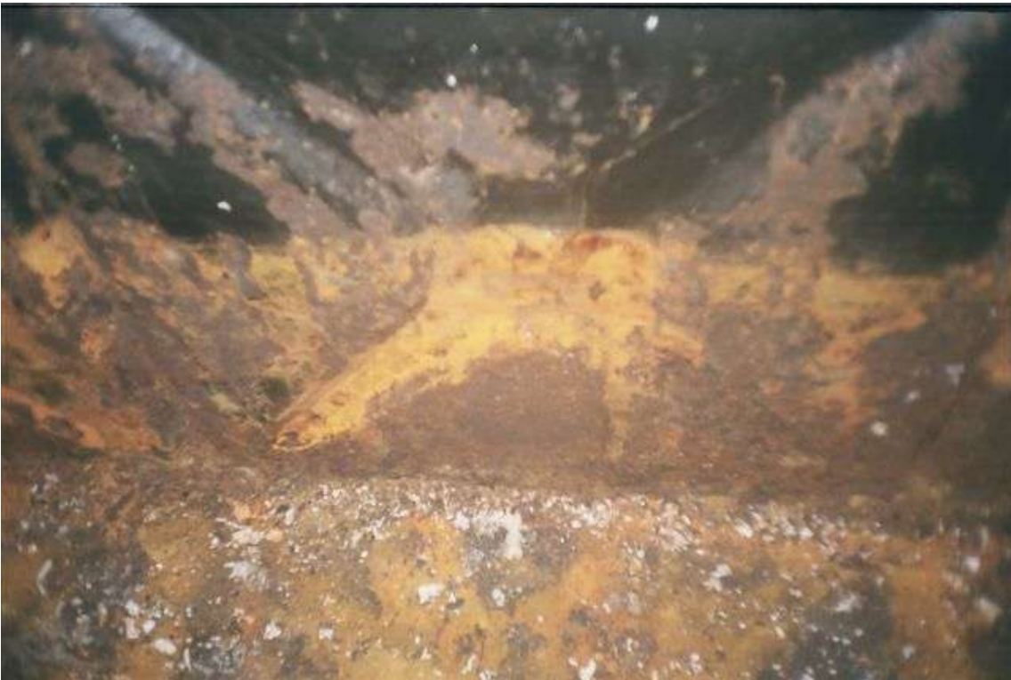
Corrosion is clearly evident as a result of water leaking behind the failed liner.
