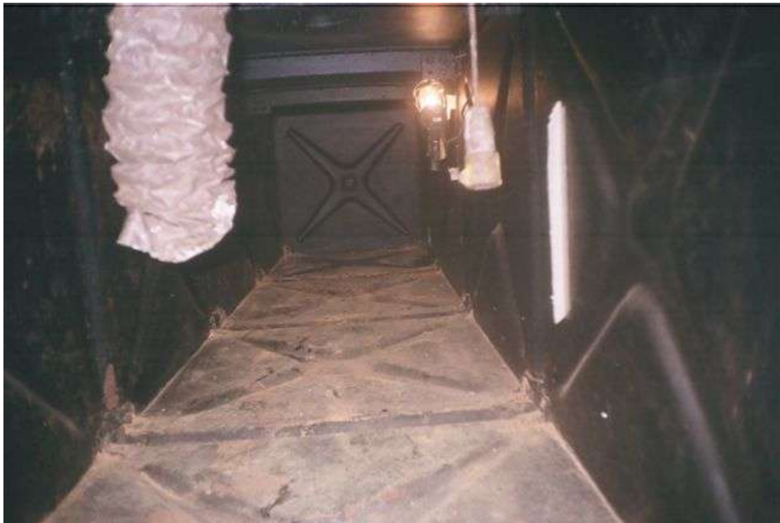
These photographs show the internal surfaces of the vessels having been drained of water with the rubber liner removed exposing the steel substrate which had been previously coated in a non (WRAS / DWI) approved bitumen paint.
