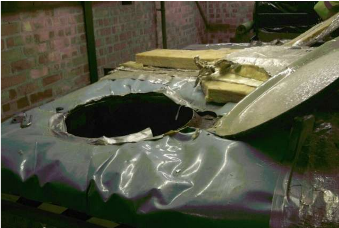
These photographs show the external of the tanks with typical access.
