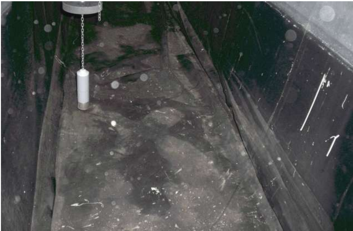
The above and following images show the internal of the structures before removal of the failed rubber liners.
