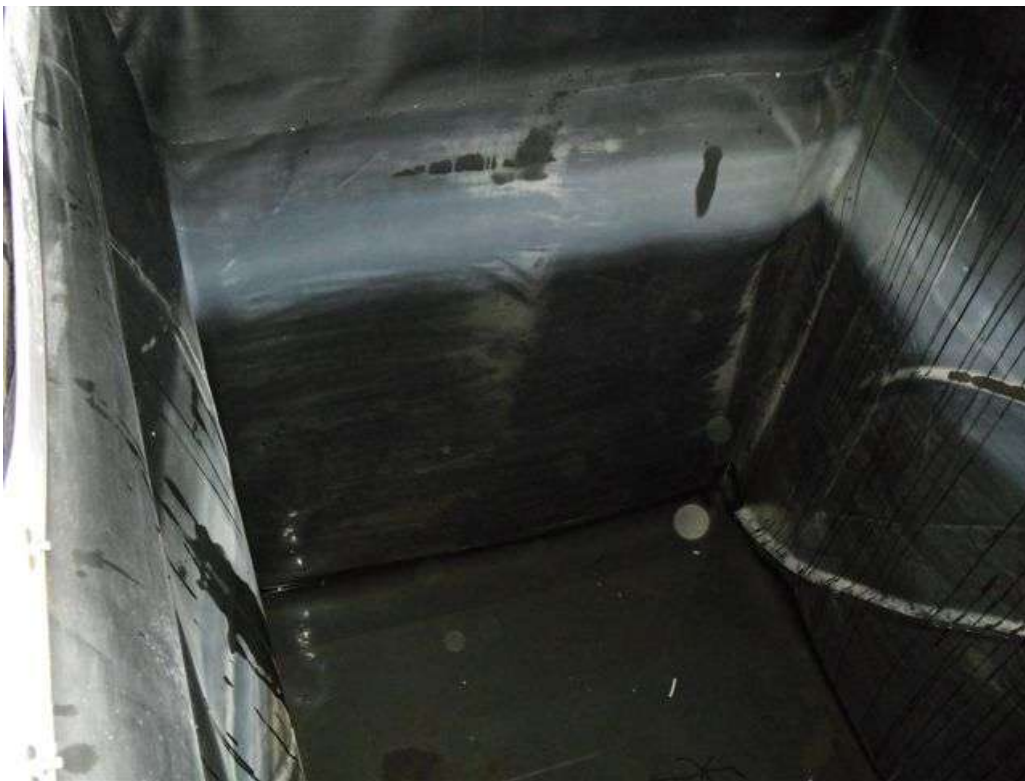
These photographs show the internal surfaces of the structure having been drained of water, but prior to the failed liner being removed and any relining work commencing.
