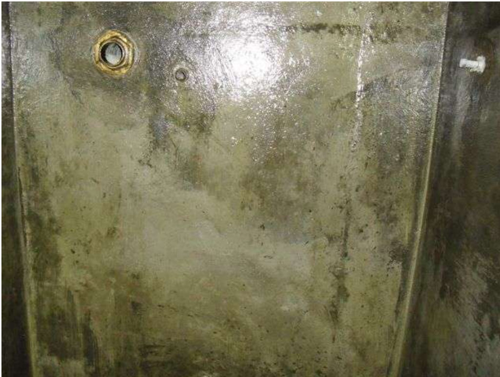
These pictures show the structure after the application of 3M Scotchkote 165PW Clear Sealer to all surfaces.
