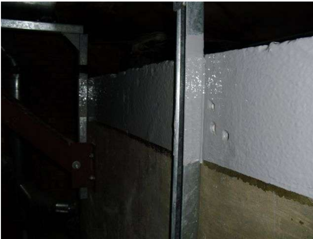
The external top and edge of the tank was also coated for additional protection.
