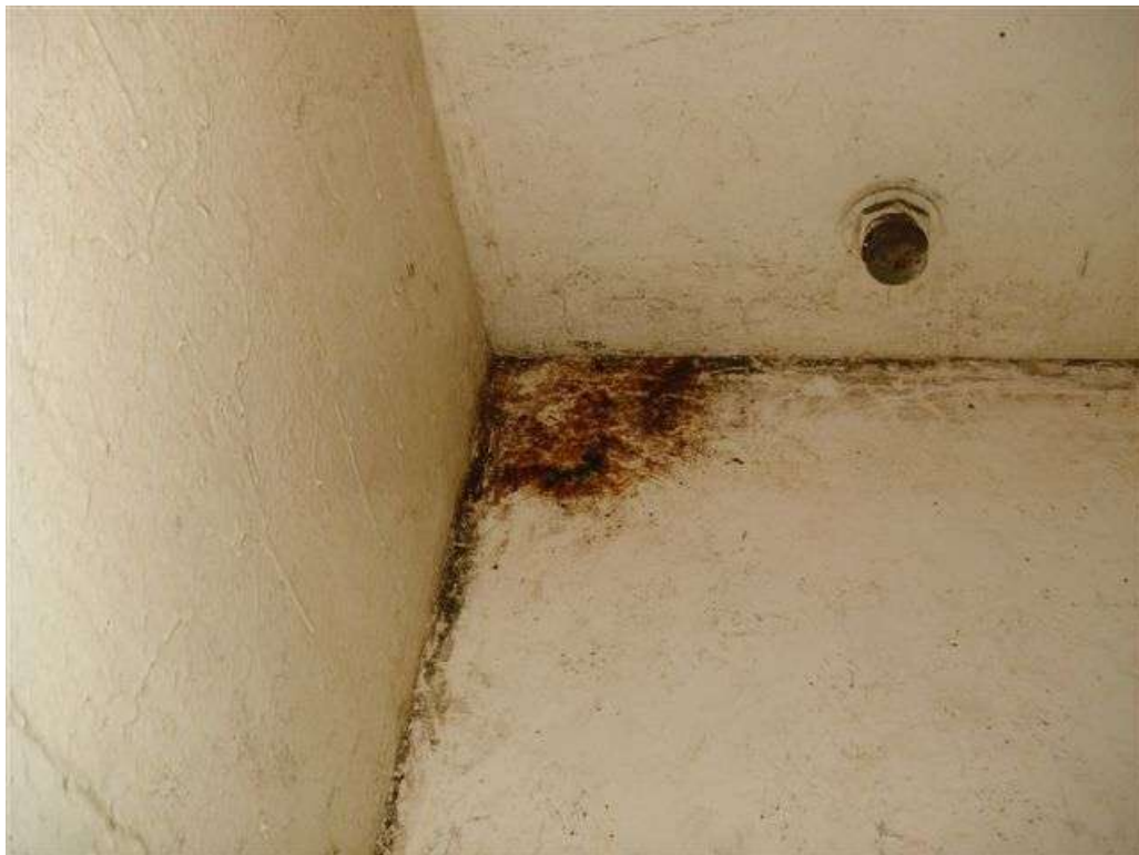
The top image highlights where the previous liner had been secured as well as remedial work to the buildings roof which had been reinforced utilising the concrete tank walls as structural supports that, in turn, had compromised the integrity of the tank.
