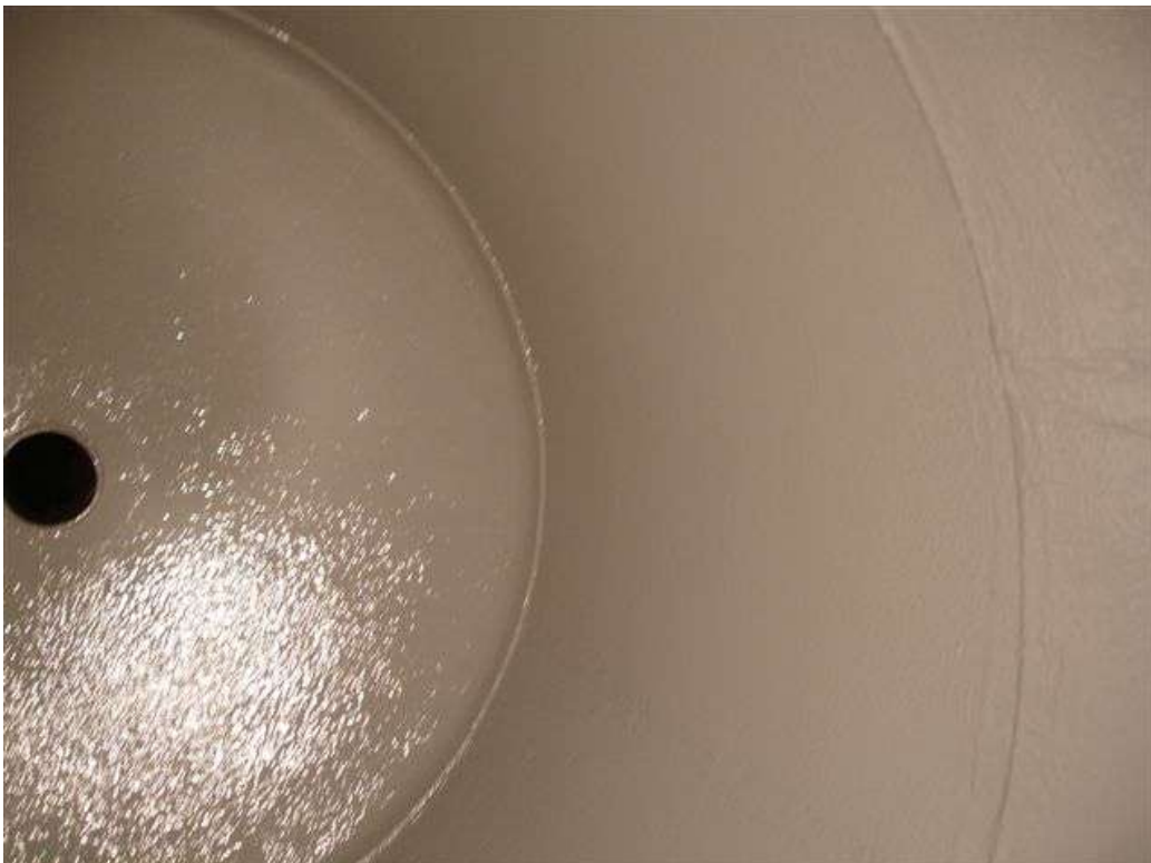
The following photographs show the final application of the 2 nd coat of 3M Scotchkote™ 165PW (grey).
