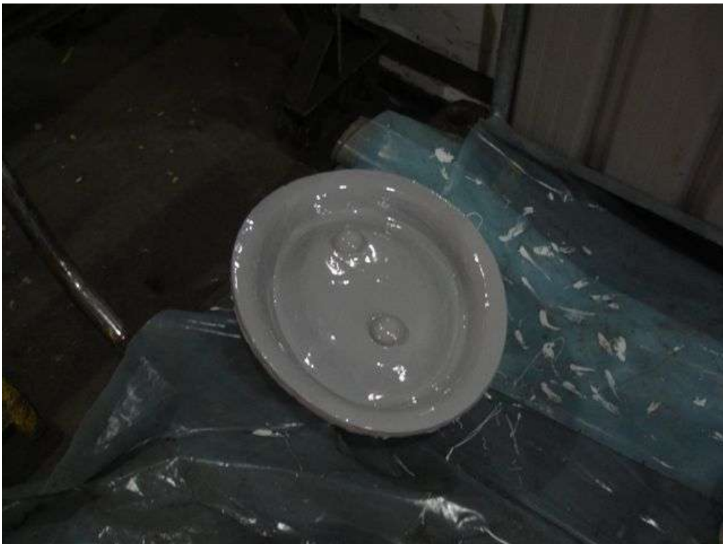
These photographs show the vessels hatches fully relined utilising 3M Scotchkote™ 165PW.
