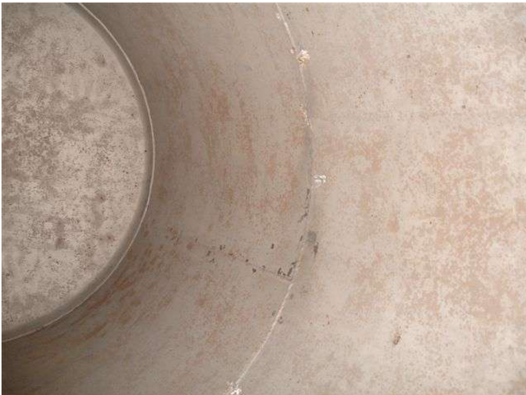
These photographs show the internal surfaces, having been prepared by COVAC Operatives using dry abrasive grit blast equipment in accordance with the accepted Standard.
