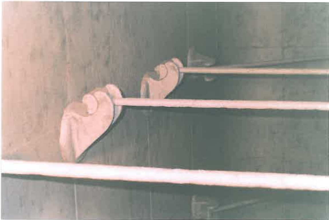
These photographs show the tank internals having been prepared to the required standard by means of dry abrasive blasting.
