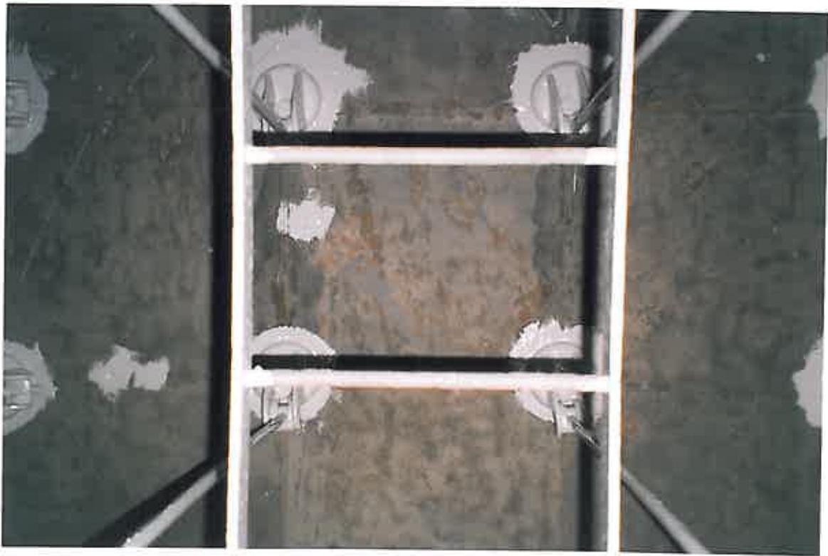
The photographs show areas such as bolt heads, struts, ladder etc, being stripe coated with 165PW by means of brush.
