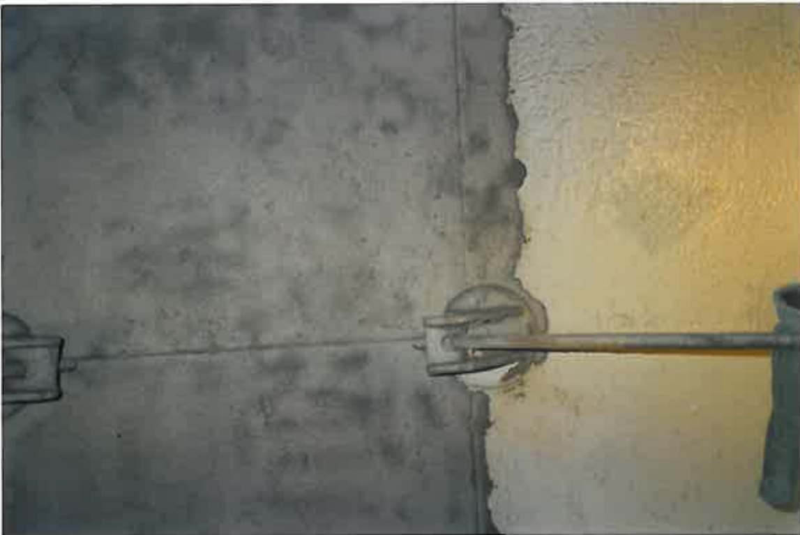
These photographs show a comparison between the previously failed coating and the standard of preparation achieved by means of dry abrasive blasting.
