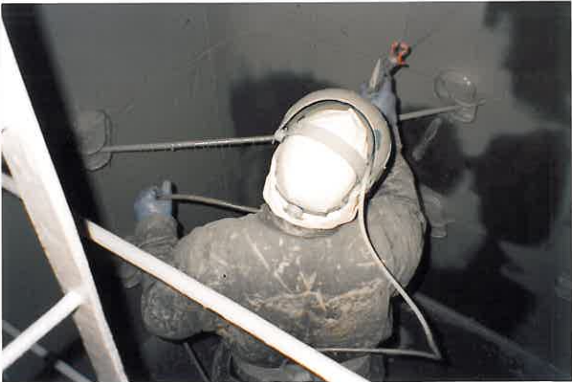
These photographs show COPON Hycote 165PW being spray applied by means of Hot Applied, Plural Component Spray Equipment.
