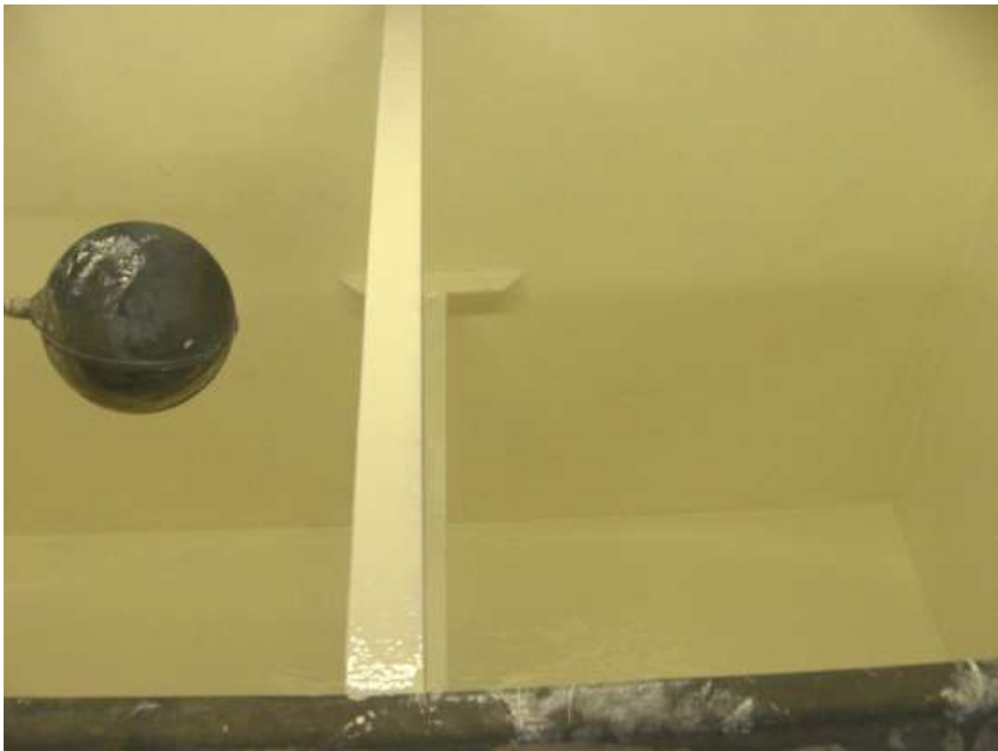
These photographs show the substrate of the tanks having received the 1 st full coat of 3M Scotchkote™ 165PW (cream) Solvent Free Polyurethane, by means of brush and roller to a nominal wet/dry film thickness of 500 Microns.
