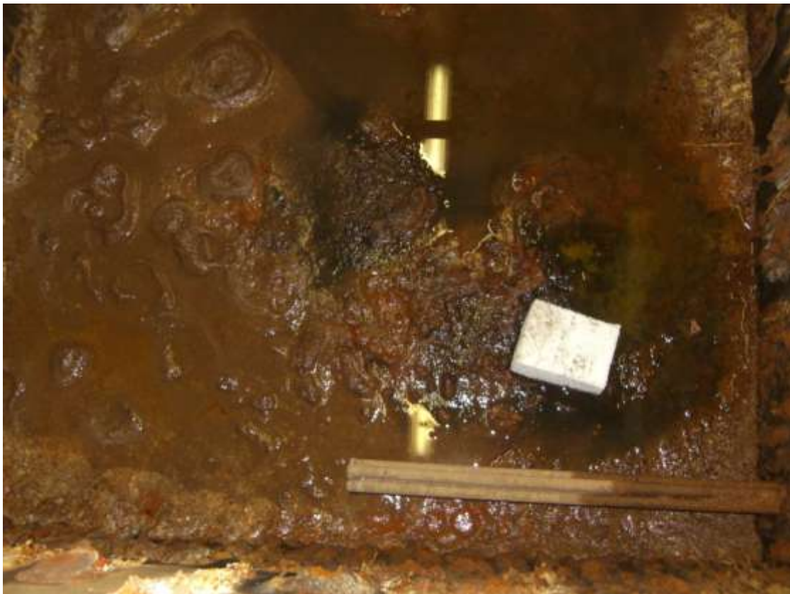
These photographs show the internal surfaces of the tanks having been drained of water and prior to any preparation works being carried out. The corrosion within the tanks is clearly evident.
