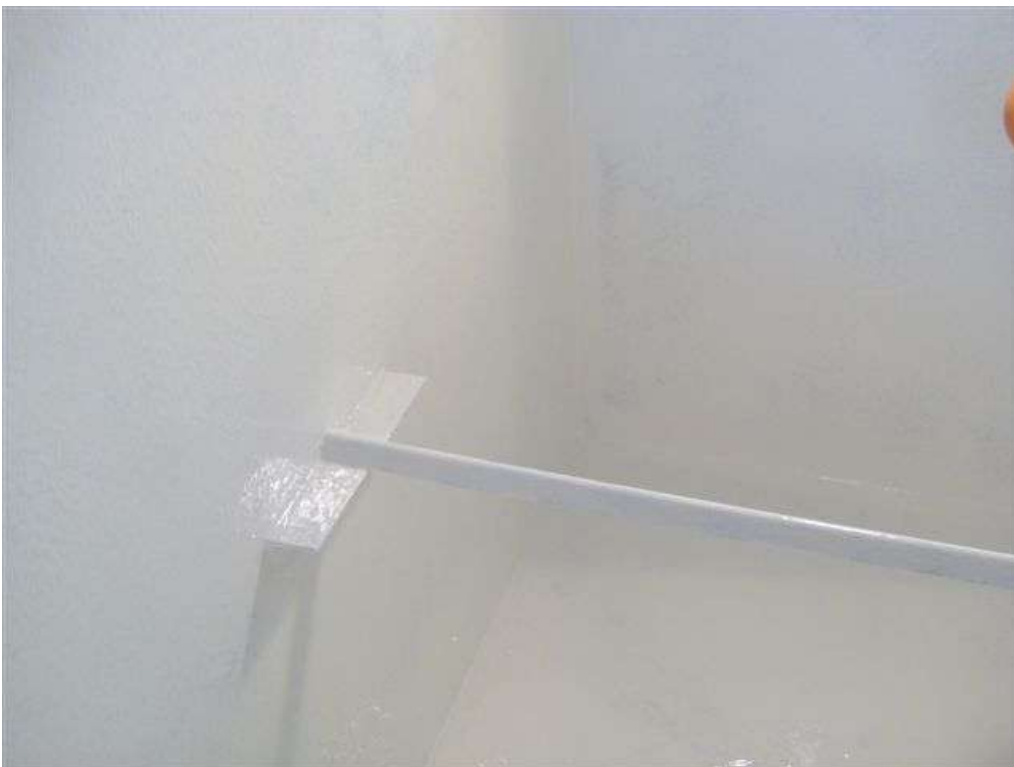
These photographs show the substrates having received the 1 st full coat of 3M Scotchkote™ 165PW (cream) Solvent Free Polyurethane, by means of brush and roller to a nominal wet / dry film thickness of 500 Microns.
