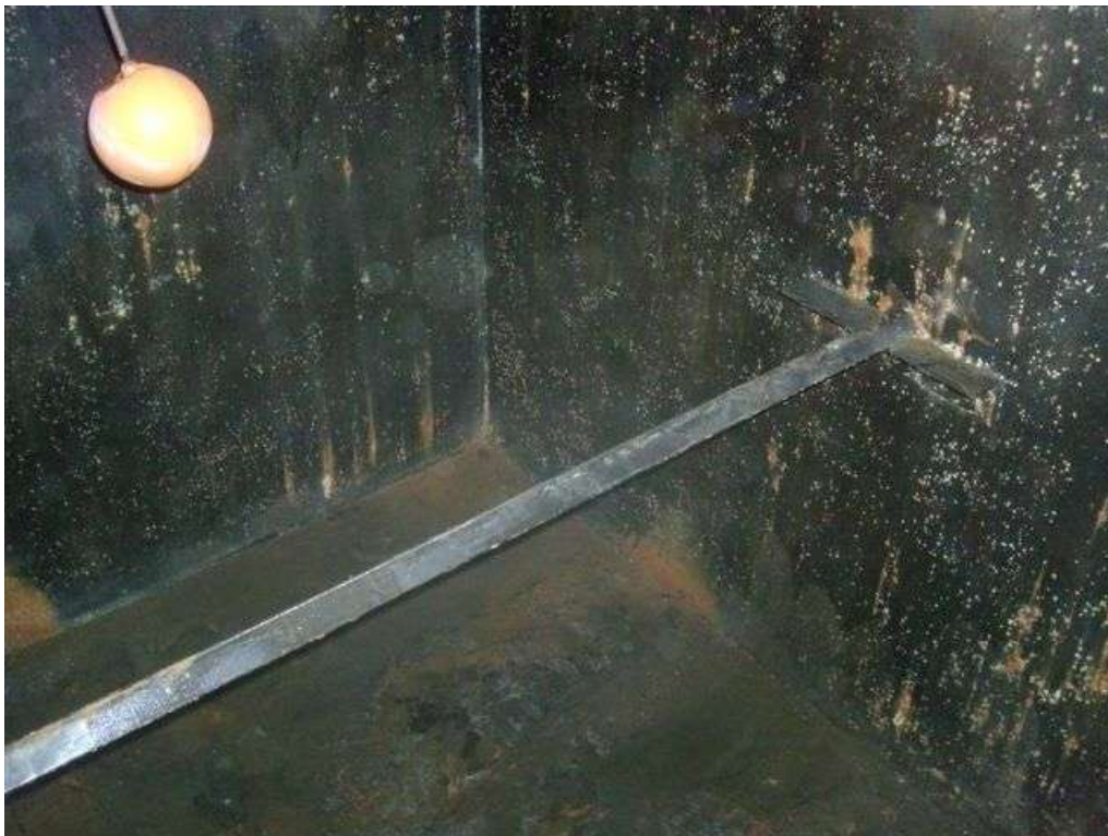
These photographs show the access to the tank and the internal surfaces of the tank having been drained of water, but prior to any work commencing, showing signs of corrosion from the non (WRAS/DWI) approved bitumastic coating.
