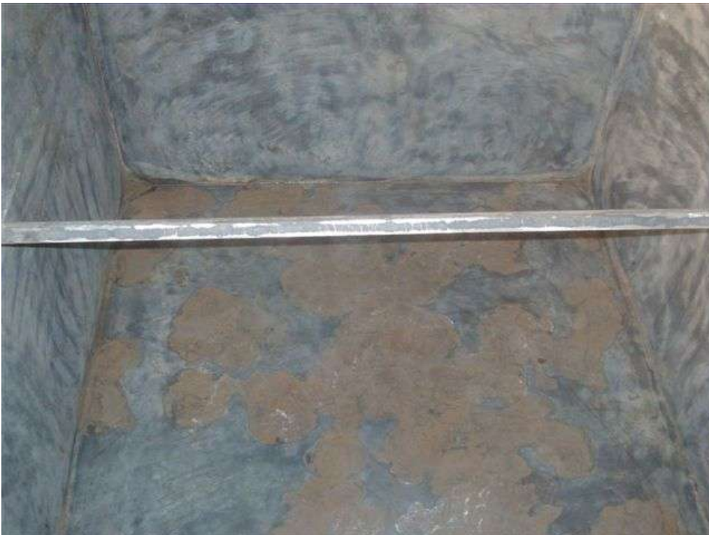
The pictures show the internal substrate after being prepared by COVAC Operatives to remove all traces of the bitumastic coating and contaminants.
