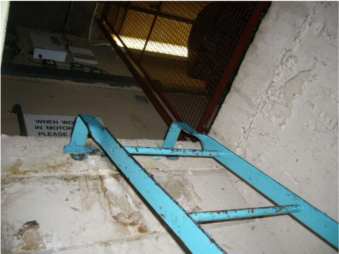
The above and following photographs show typical access to the concrete water retaining structures.
