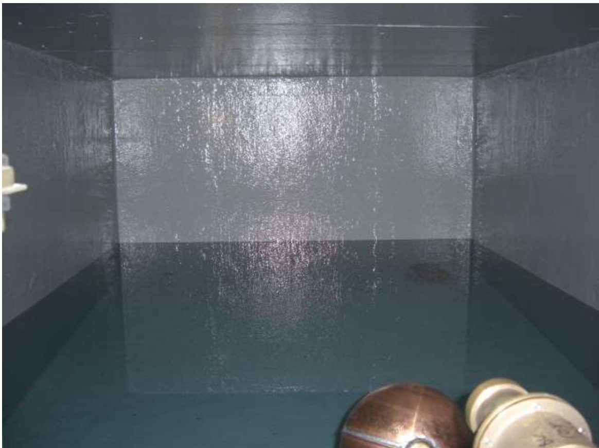
All intricate areas were again 'stripe coated' for a second time followed by the final application of the 2 nd coat of 3M Scotchkote™ 165PW. These images show the tanks fully relined and refilled with potable water.
