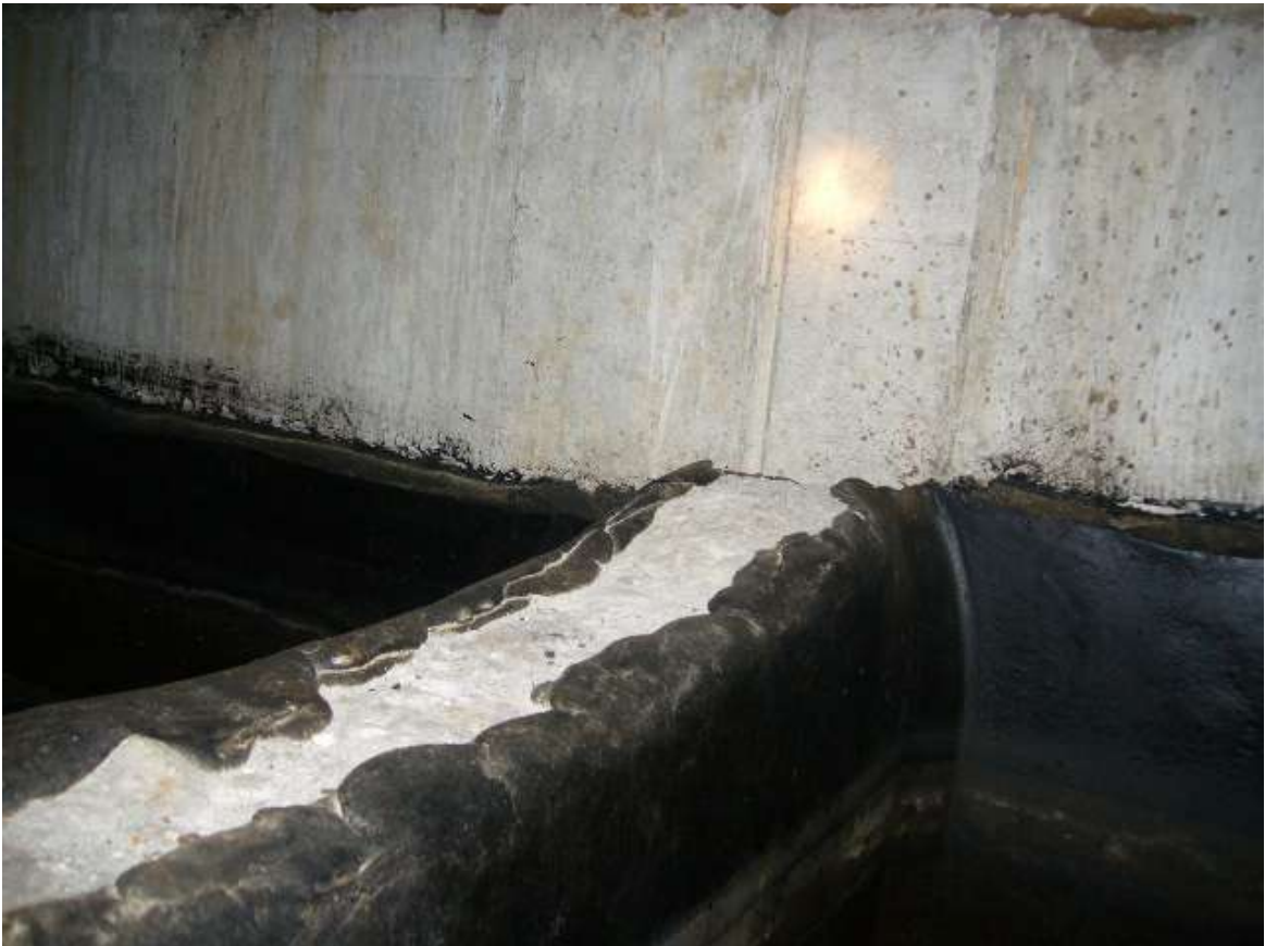
These images show the asphalt coating that was previously applied up to the water line. Above the water line and the roof slab was bare concrete.
