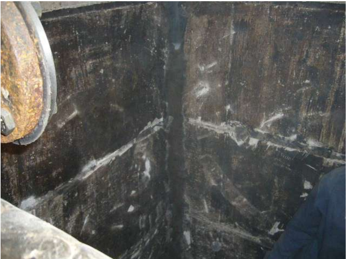
These photographs show the internal surfaces whilst being prepared by COVAC operatives to raise a suitable surface profile.
