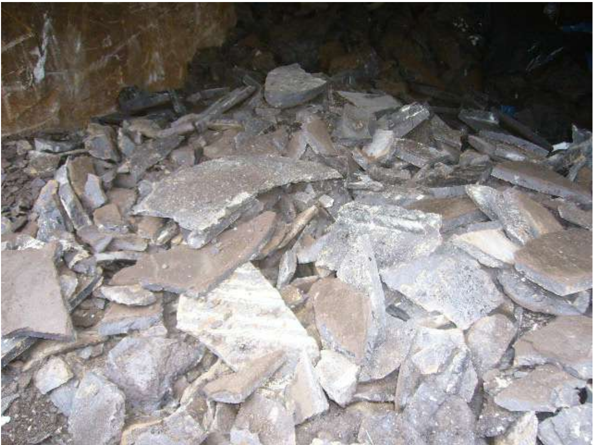
These images show the thickness and quantity of the asphalt coating removed from the internal substrate of the tanks.
