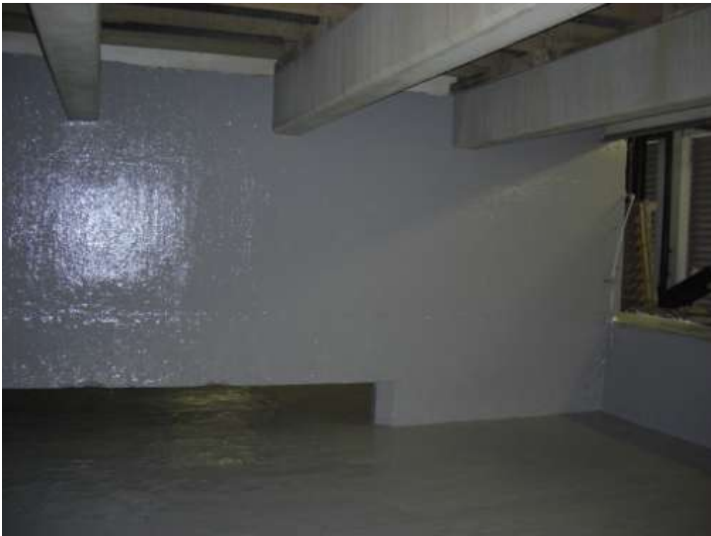
These images show the second coat of 165PW (grey) prior to the external louver doors being replaced.
