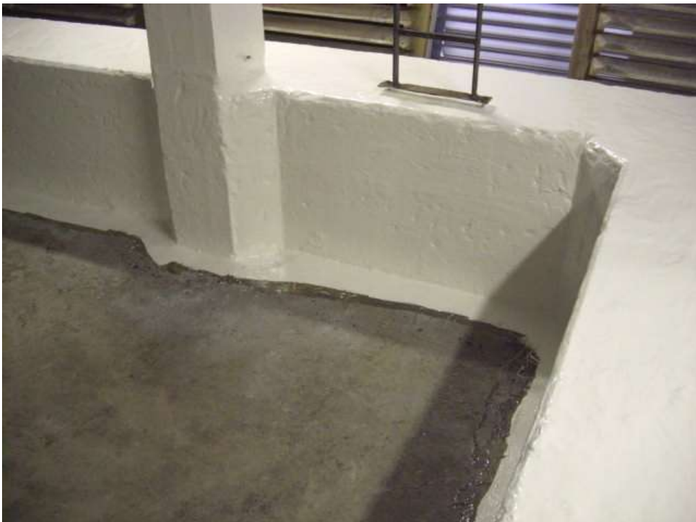
Images showing the first coat of 3M Scotchkote 165PW (cream) being applied.
