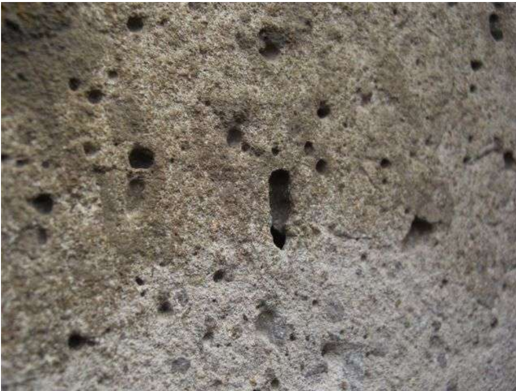
These 'close up' images show the blow holes exposed within the concrete.
