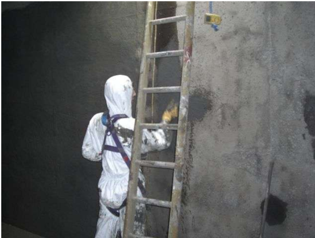
These photographs show the DWI Approved Cementitious Polymer Modified, Screed and Pore Filler being applied to the concrete surface which was allowed to cure and dry completely for the specified period.
