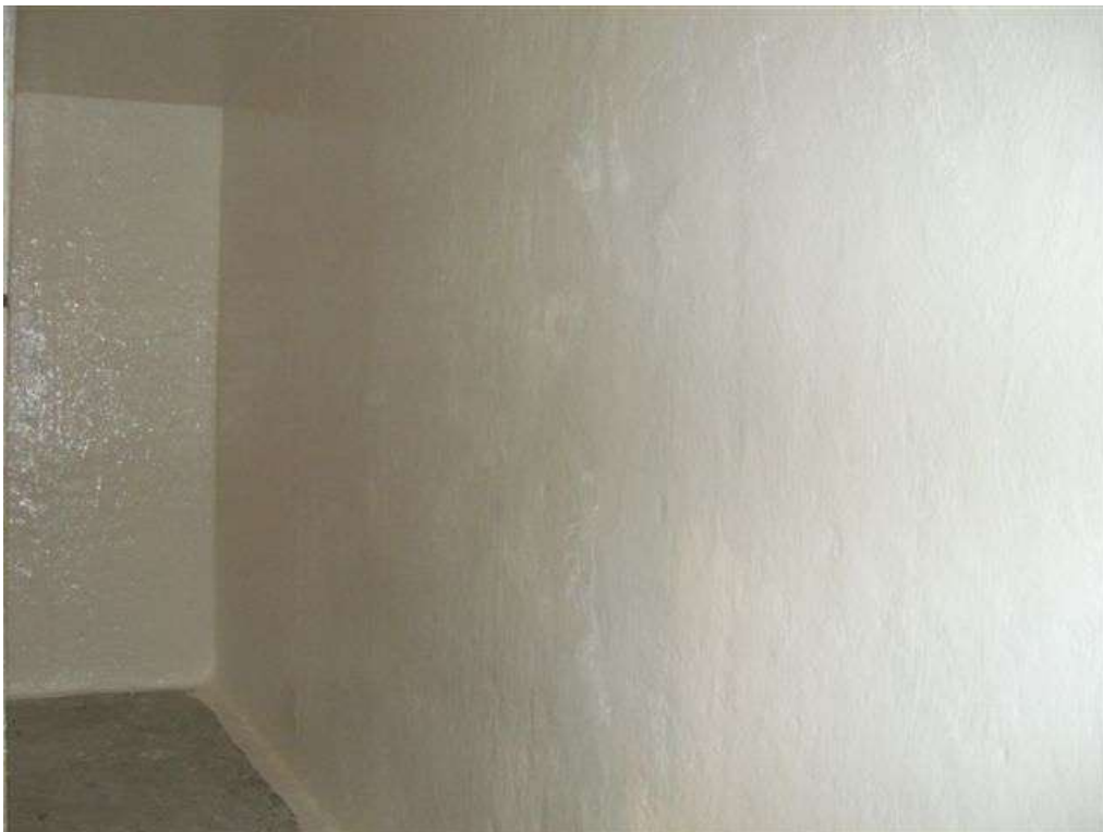
All joints, seams and intricate areas were initially 'stripe coated'. These photographs show the substrates during the 1 st full coat of 3M Scotchkote™ 165PW (cream) Solvent Free Polyurethane.
