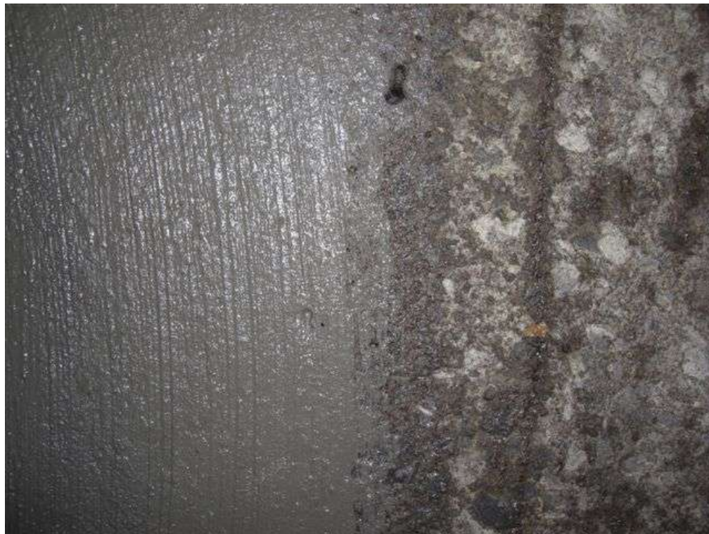
These images show the comparison between the prepared concrete and the application of the DWI Approved Cementitious, Polymer Modified, Screed and Pore Filler.
