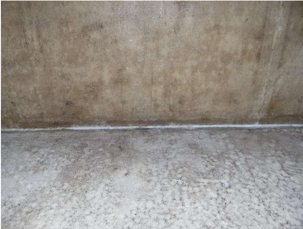
These photographs show the internal surfaces of the tanks having been drained of water, but prior to any work commencing.
