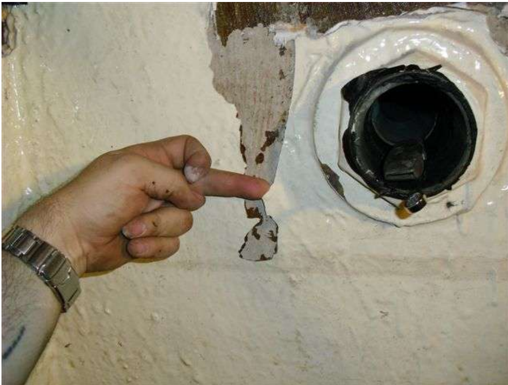
The coating was clearly de-laminating from the concrete substrate.
