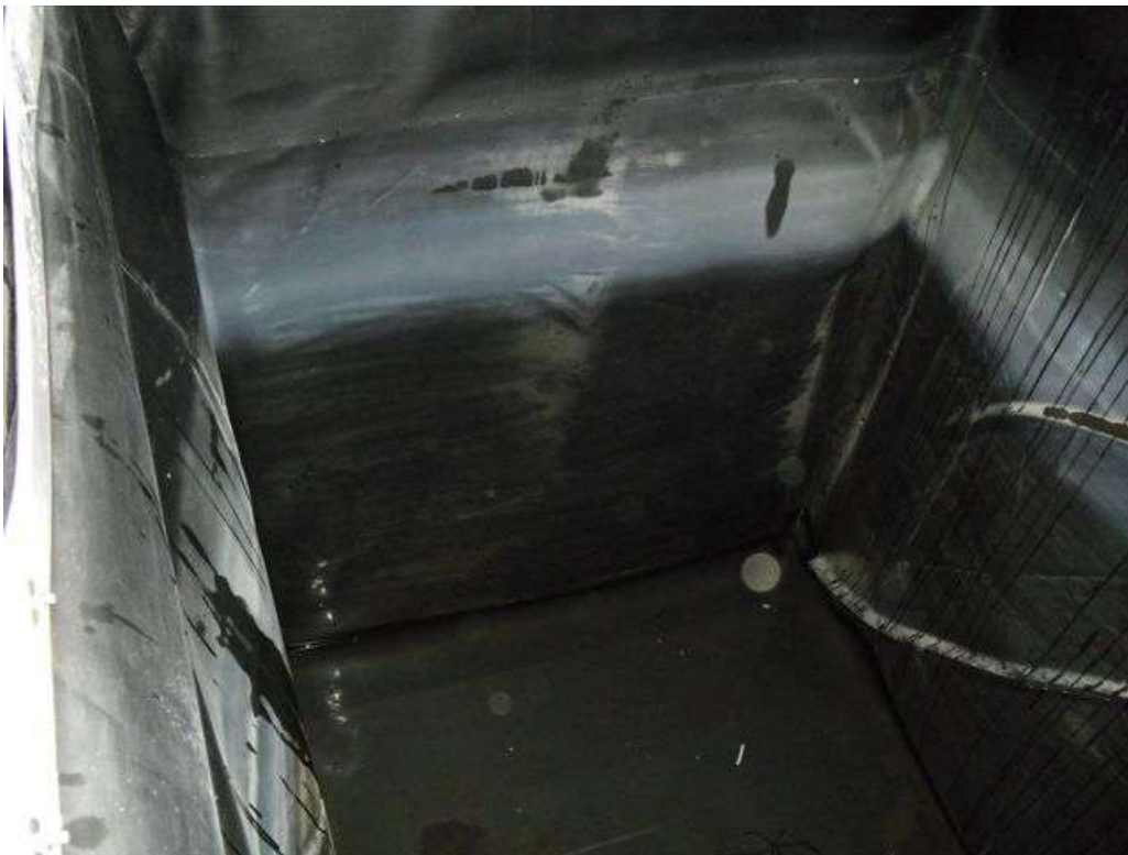
These photographs show the internal surfaces of the structure having been drained of water, but prior to the failed liner being removed and any relining work commencing.
