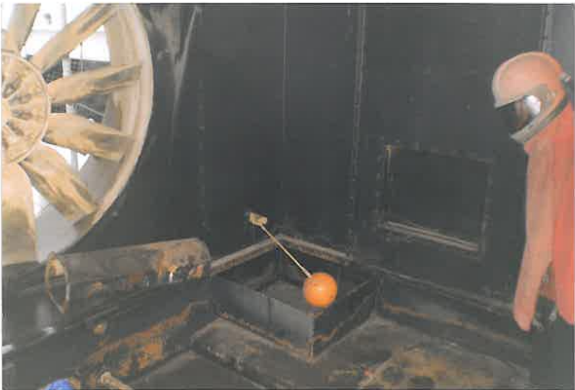
These photographs show the internal substrate of the tower and the severity of the corrosion. The previous coating system, which had reached the end of its useful life showing due to sub-film corrosion, low film build and general deterioration.
