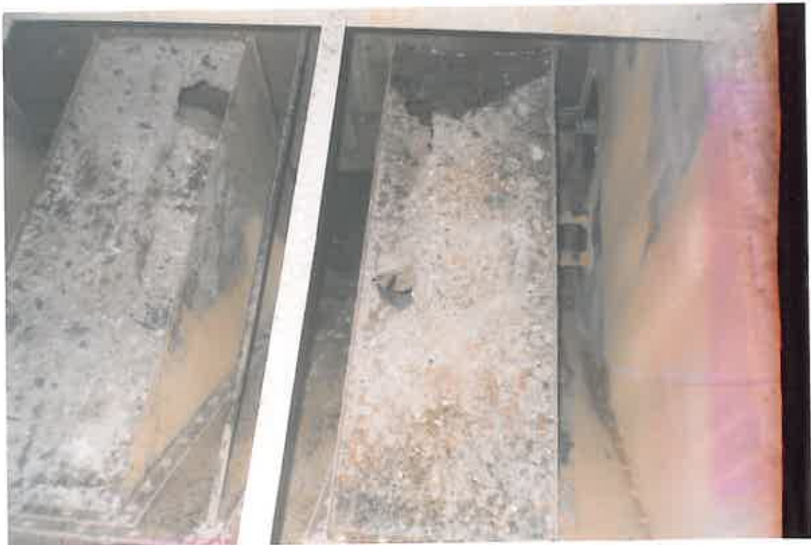
On initial inspection severe corrosion was found to be apparent on numerous components, which were removed & subsequently replaced once the coating process had been completed.
