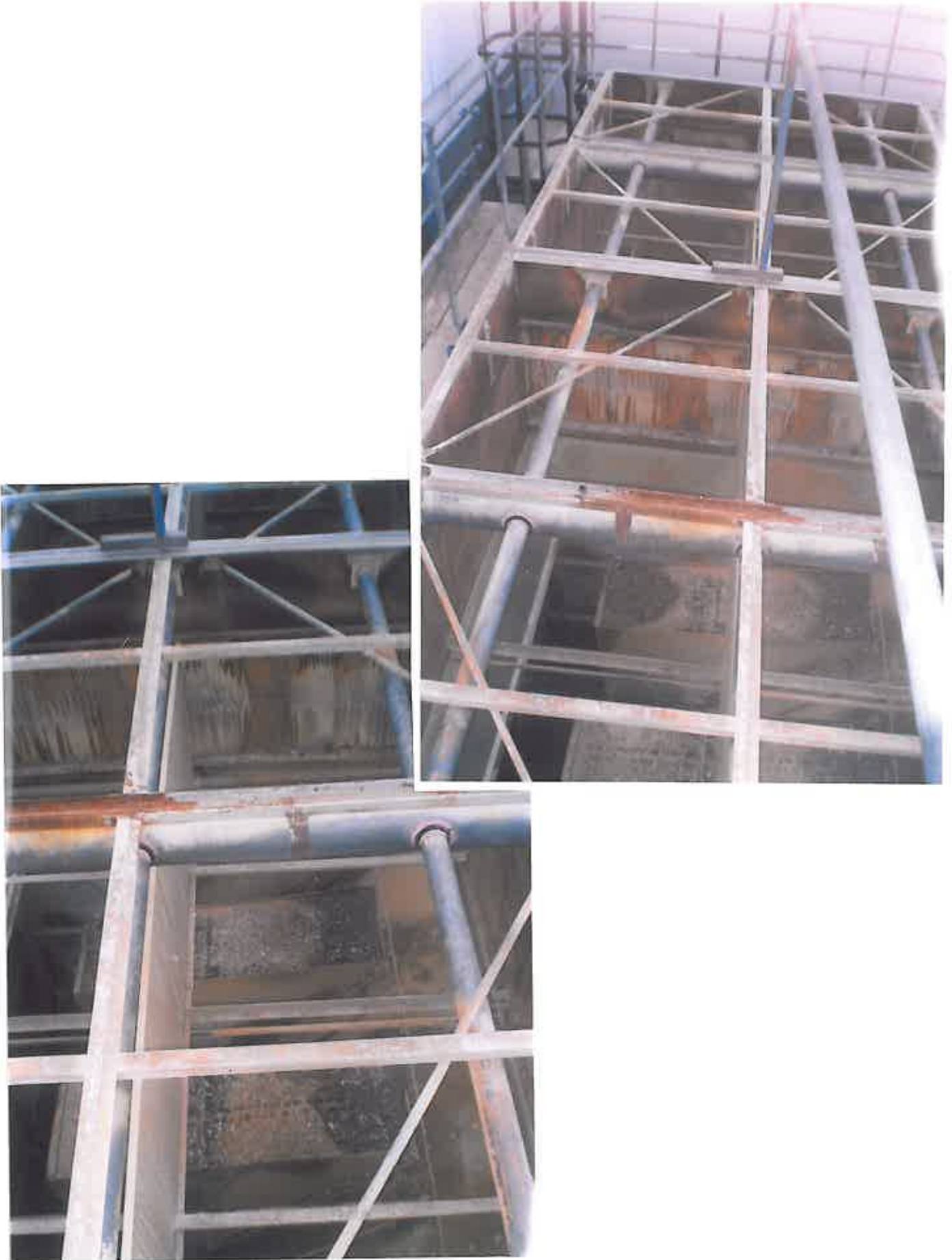
The above photographs show the internal substrate of the 2 No. Towers prior to any preparation work involved in removing all of the existing failed non flexible epoxy coating.
