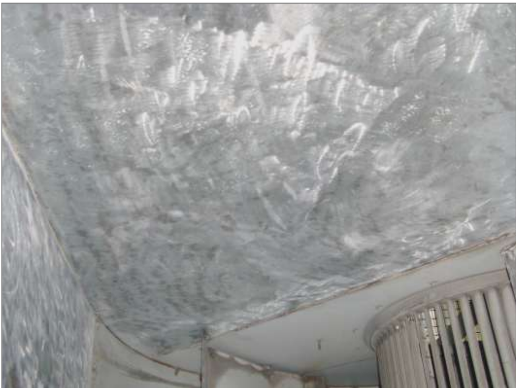
These pictures show the substrate following preparation by COVAC Operatives using Tungsten Carbide Scabblatex Units and Scrapers in accordance with ISO 8501-1:2007.
