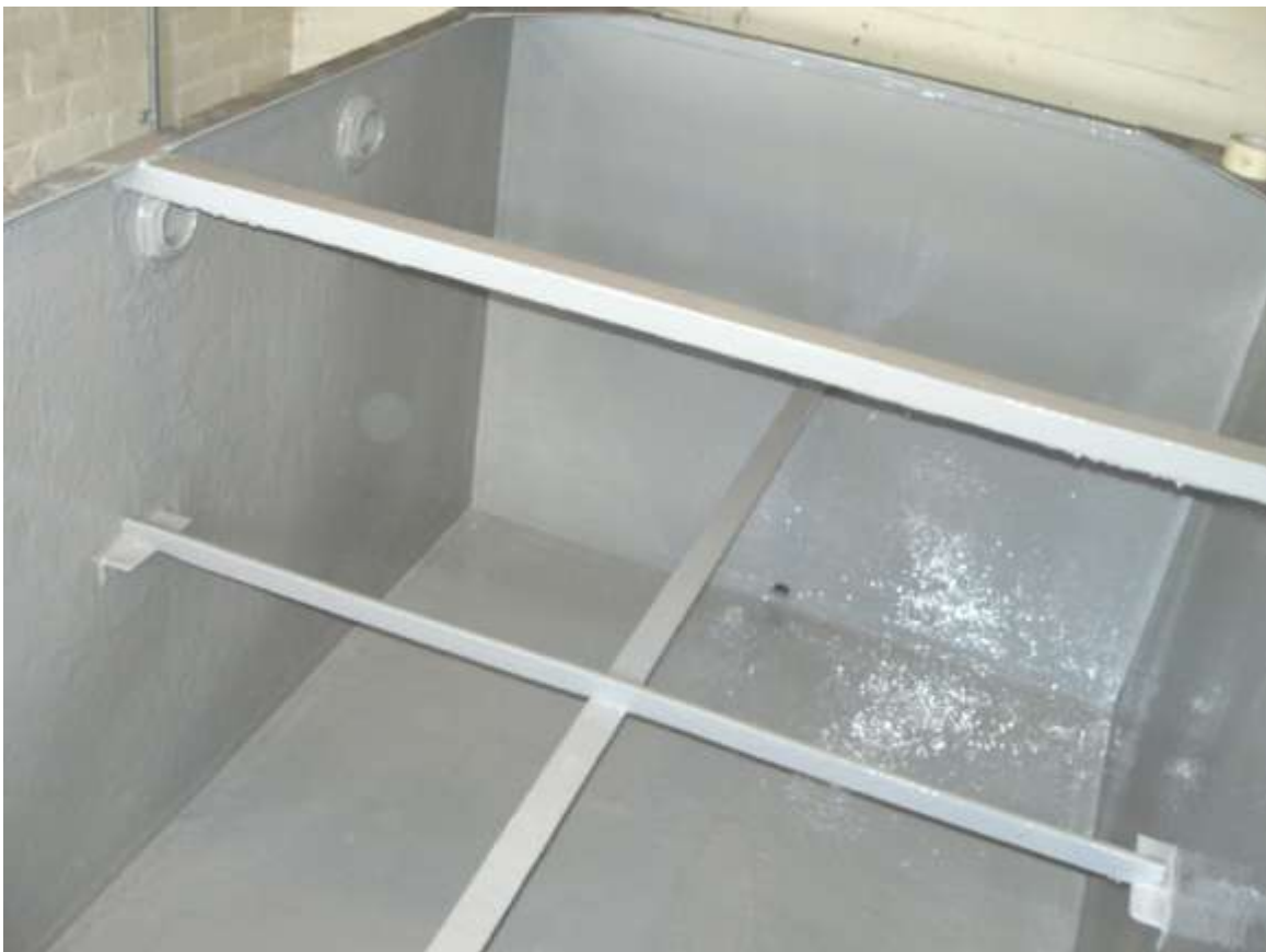
The following photographs show the final application of the 2 nd coat of 3M Scotchkote™ 165PW (grey) in order to achieve a total, nominal dry film thickness of 1000 Microns (1mm), and between 1500-2000 Microns (2mm) over all stripe coated areas.
