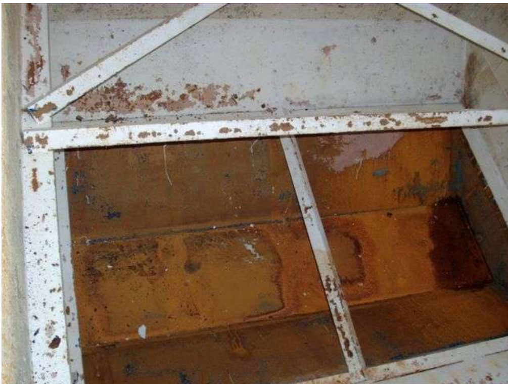
These photographs show the internal surfaces of the tank having been drained of water, but prior to any work commencing.
