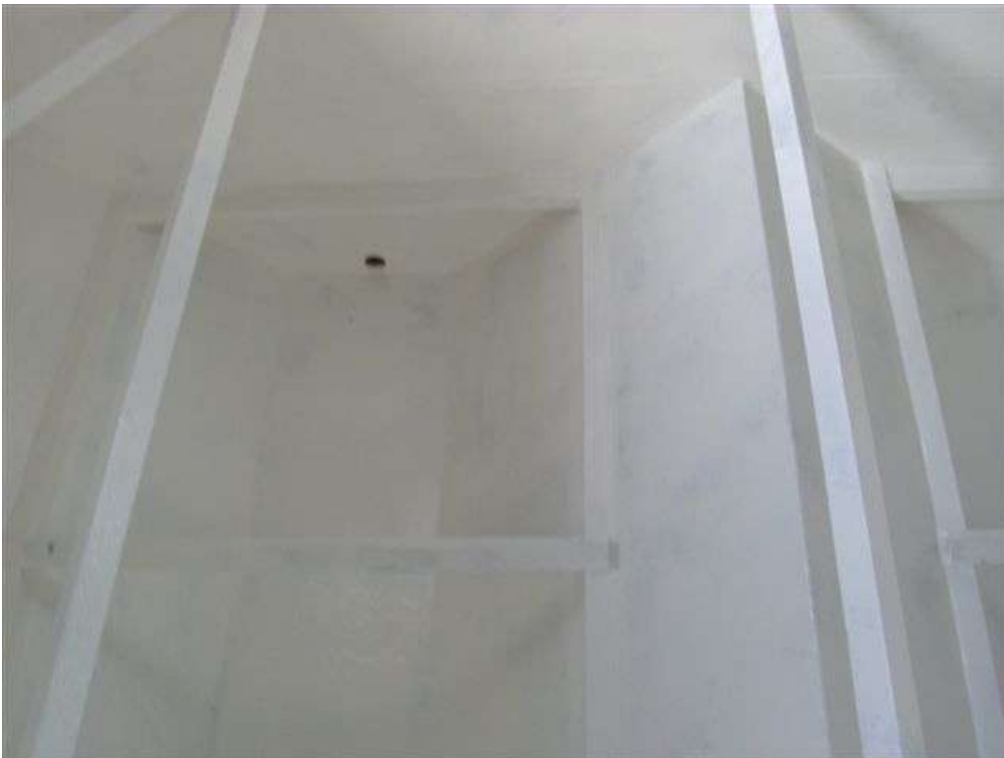
These photographs show the substrates having received the 1 st coat of 3M Scotchkote™ 165PW (cream) Solvent Free Polyurethane.
