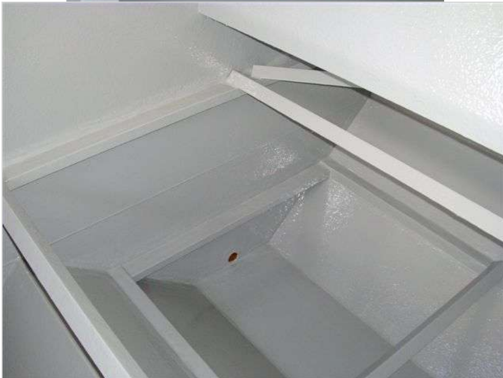
All intricate areas were again 'stripe coated' for a second time. The following photographs show the full and final application of the 2 nd coat of 3M Scotchkote™ 165PW (grey).
