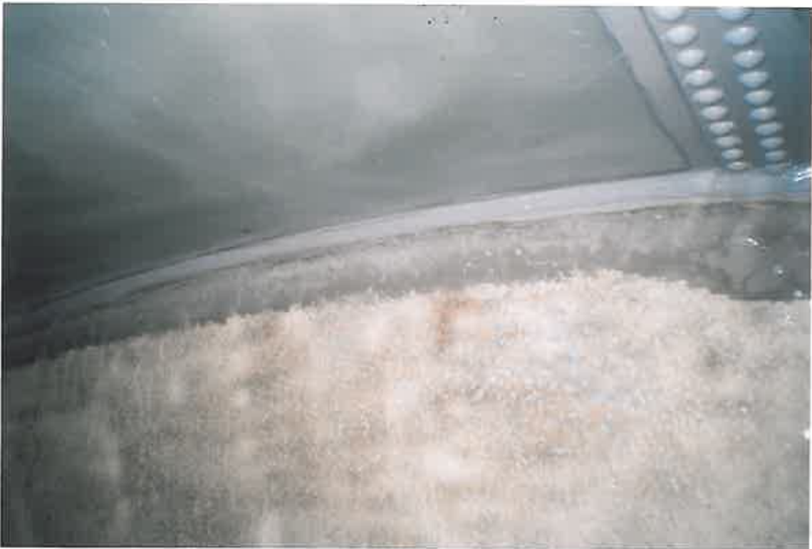
Concrete repairs were carried out on the floor areas, where required, using a cementitious epoxy repair mortar.
