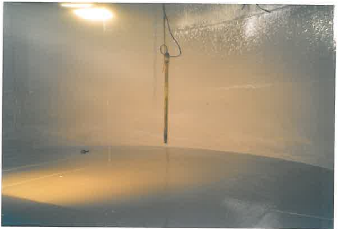
These photographs show the internals of the tank completely re-lined with COPON Hycote 165PW applied to a nominal dft of 1000 Microns (1mm).
