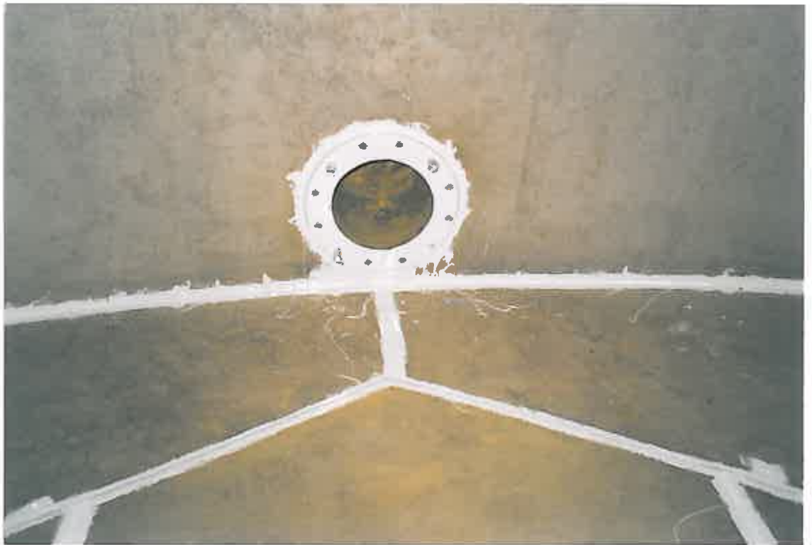
These photographs show all the jointed areas, sharp edges, ladder, etc. having been 'stripe' coated by brush with COPON Hycote 165 PW.
