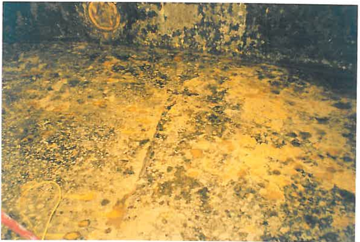
These photographs show the tank drained of water and prior to preparation works. The photographs clearly show that the existing Bitumen part had approached the end of it's useful life due to excessive sub-film corrosion, low-film build and general deterioration.
