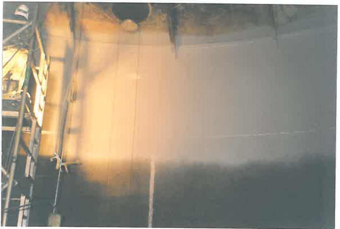
These photographs show the application of COPON Hycote 165PW to all prepared, internal surfaces of the tank by means of Plural Component 'Hydra-Cat' Spraying Equipment.
