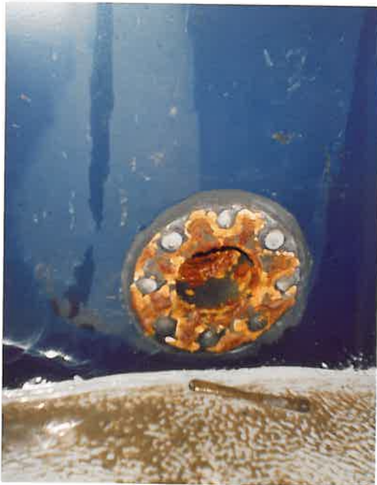
These pictures show the drain hole and the lower access hatch, which had been removed, making entry and egress easier throughout the project.
