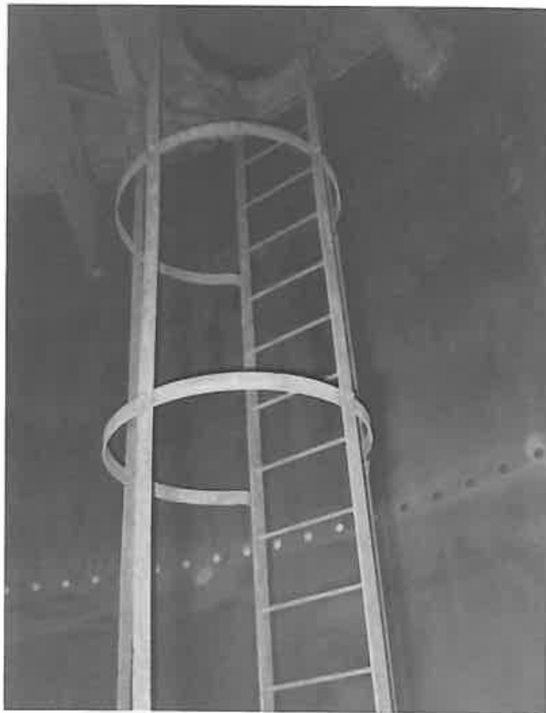
These photographs show all internal surfaces of the tank having been prepared in accordance with the accepted SA 2.5 / BS7079 standard by means of dry abrasive blasting techniques.
