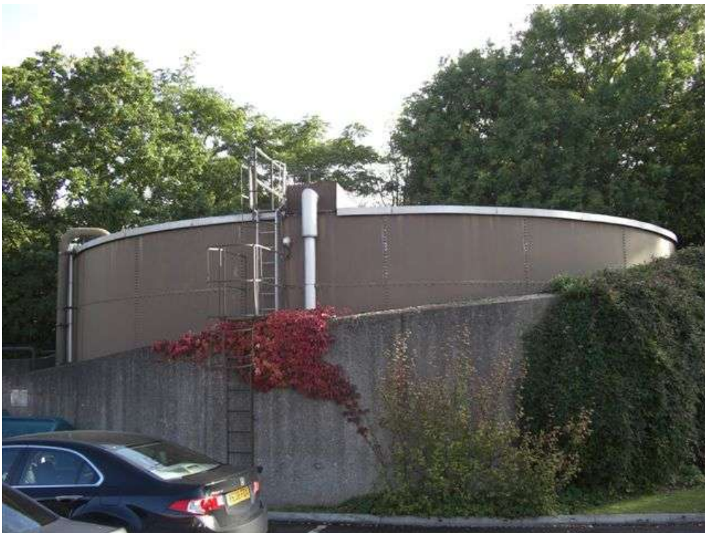
These photographs show the external of the tank prior to any work commencing.
