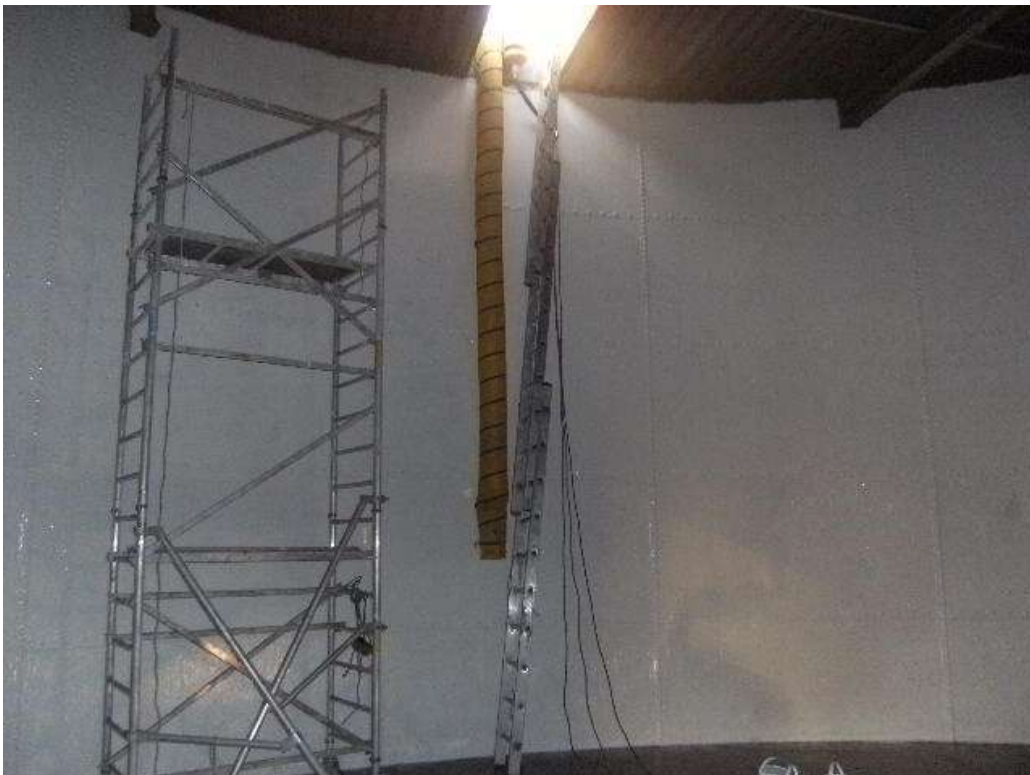
All seams, joints, bolts etc were initially 'stripe coated' to ensure all intricate areas were coated prior to the 1 st full coat of 3M Scotchkote™ 165PW Solvent Free Polyurethane. These photographs show the steel substrate having received the 1 st full coat of 3M Scotchkote™ 165PW (cream) Solvent Free Polyurethane, by means of brush and roller
