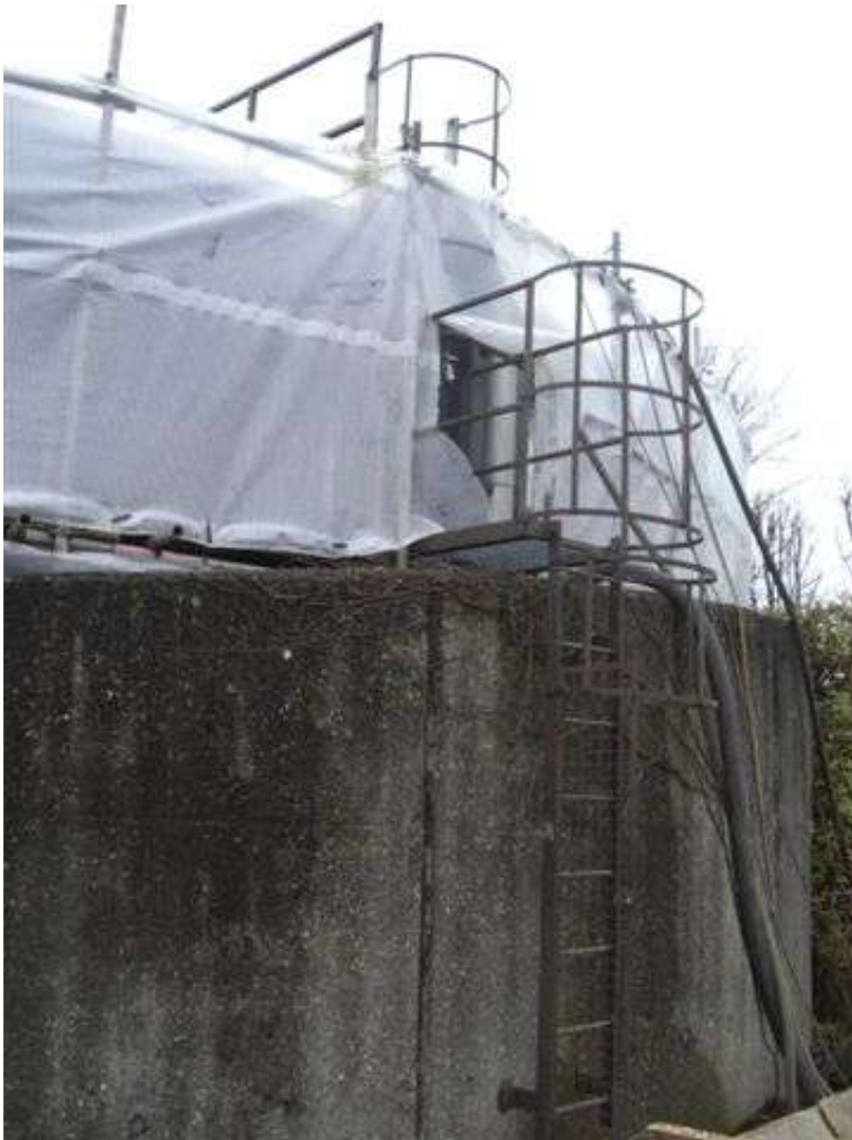
These photographs show the structure sheeted off to protect against inclement weather and also access to the structure.
