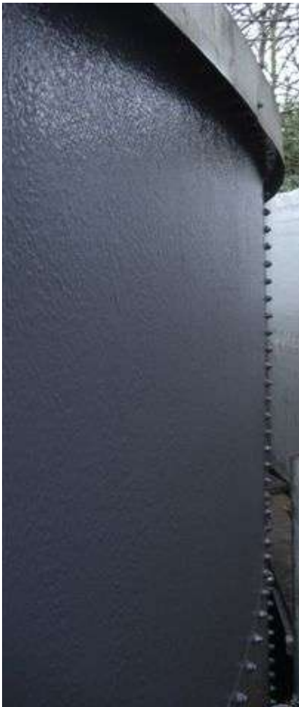
These photographs show the external substrate having received the 1 st coat of 3M Scotchkote™ 152LV.
