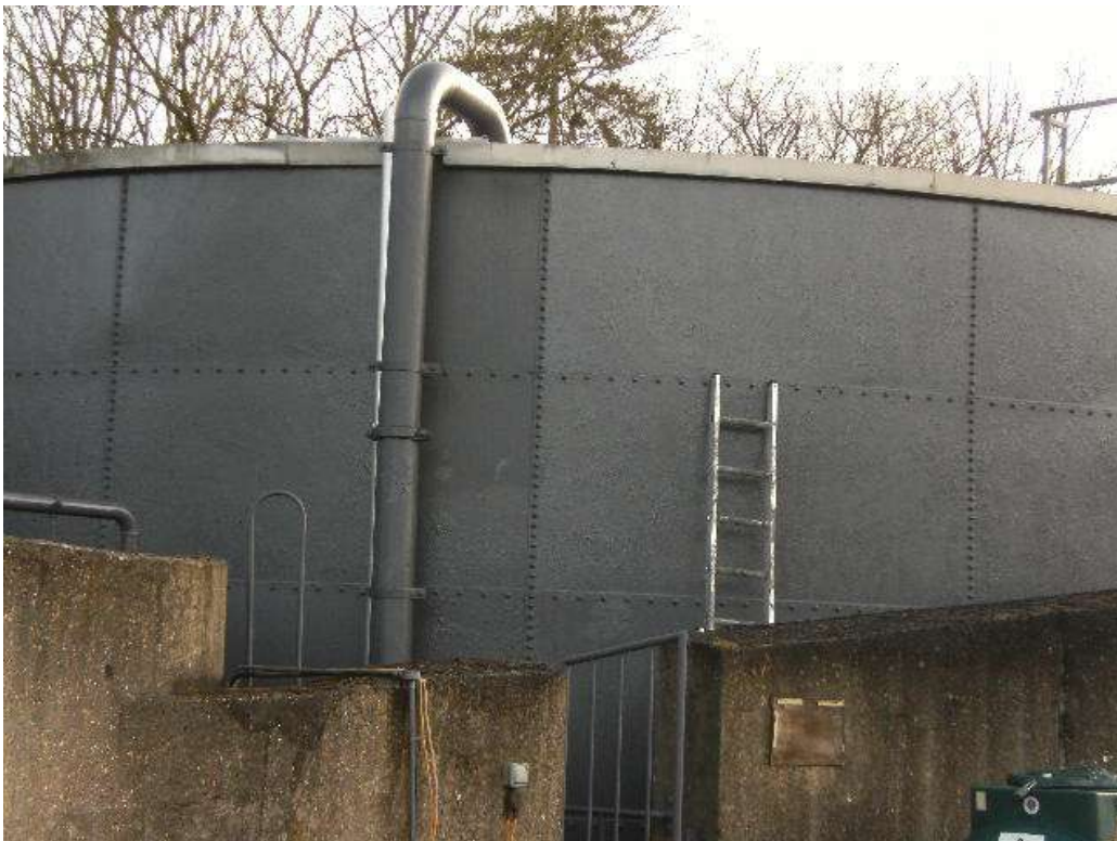
These photographs show the external substrate having received the final coat of 3M Scotchkote™ 152LV.
