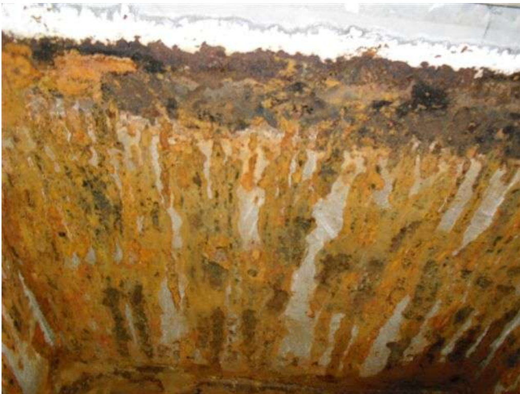
These photographs show the internal surfaces of tank #2 having been drained of water, but prior to any work commencing. As with tank #1, severe corrosion is evident resulting in holes in the substrate, particularly at the waterline.
