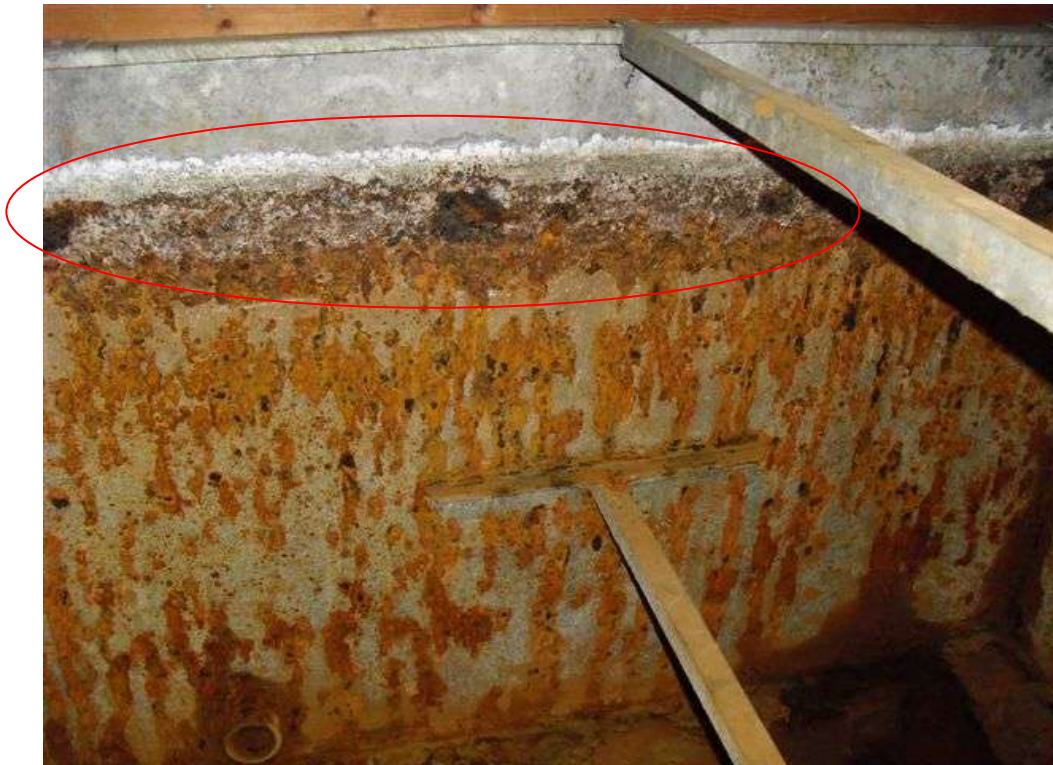
Holes in the substrate at the waterline as a result of the severe corrosion can be seen.
