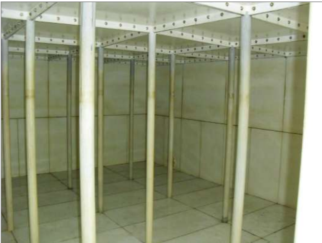
These photographs show the internal surfaces of the Structure having been drained of water, but prior to any work commencing.
