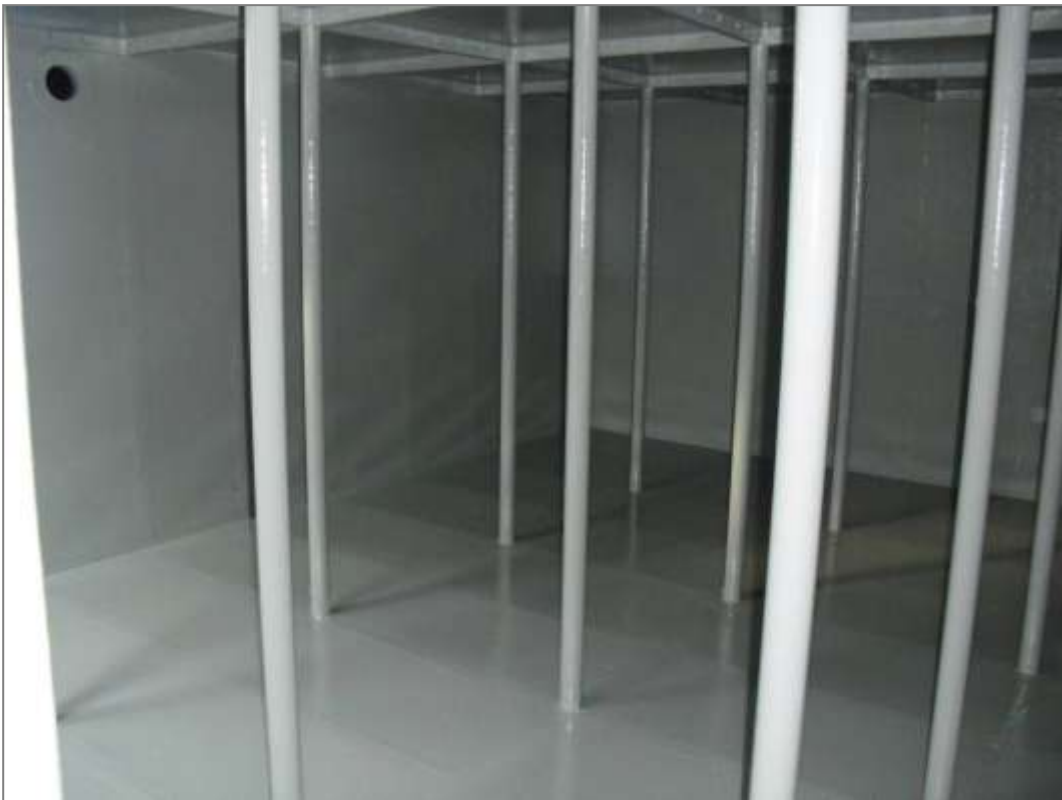
These photographs show the internal surfaces following the full coat of 3M Scotchkote™ 165PW Solvent Free Polyurethane.
