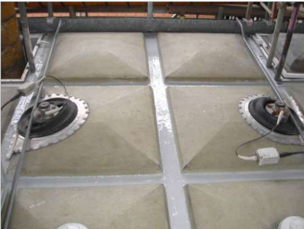
These images show the external joint once coated with 3M Scotchkote 165PW.
