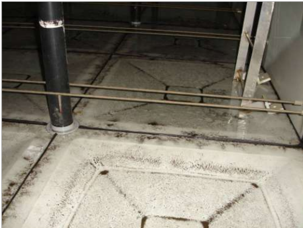
These photographs show the internal surfaces of the structure, having been drained of water and prior to relining work commencing.
