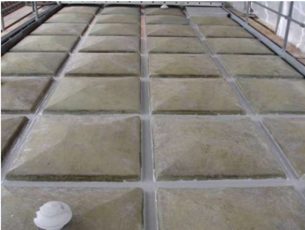
These images show the external joint once coated with 3M Scotchkote 165PW.
