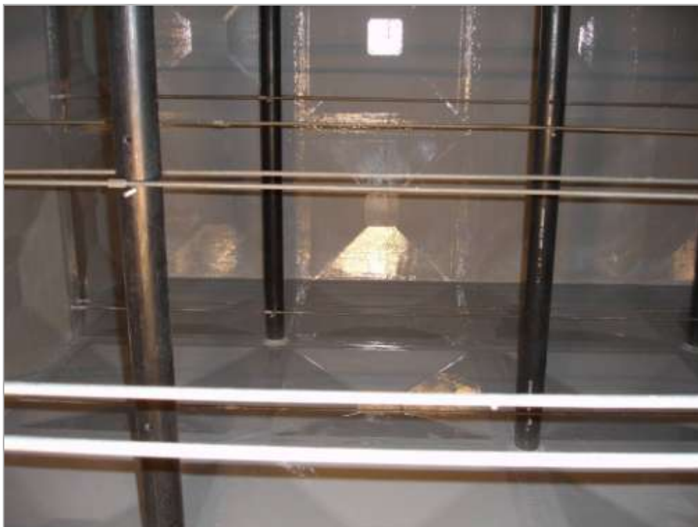
The following photographs show the internal of the structure after being fully coated with 3M Scotchkote 165PW (grey) Solvent Free Polyurethane, by means of plural component spray equipment.
