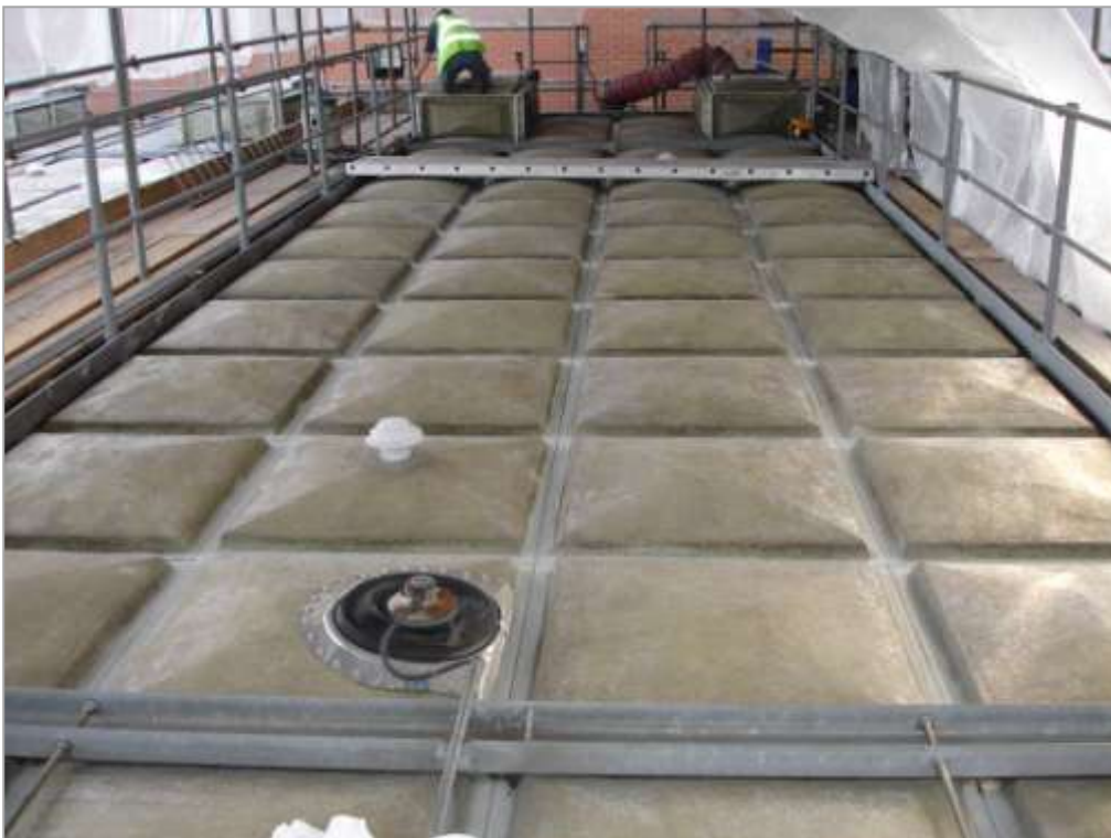
These pictures show the external roof joints of the structure being prepared by COVAC Operatives in order to raise a suitable surface profile to promote optimum adherence of the 3M Scotchkote™ 165PW system.
