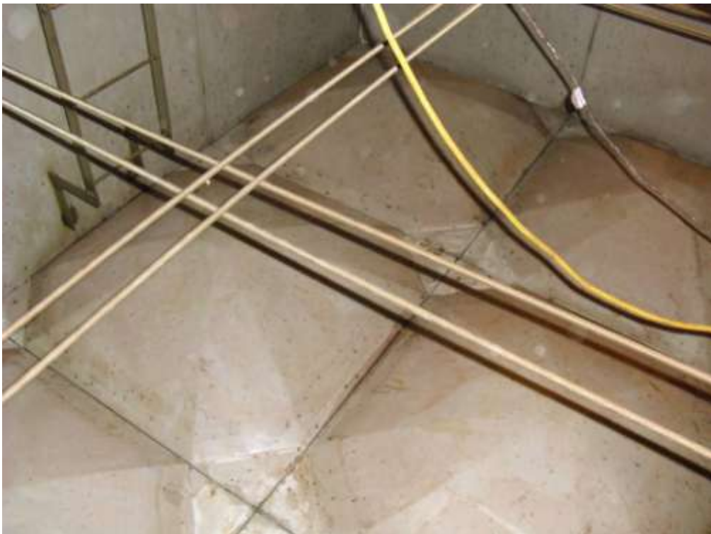
These photographs show the internal surfaces of the tank having been drained of water and prior to relining work commencing. Black spore fungi can be clearly seen over much of the substrate.
