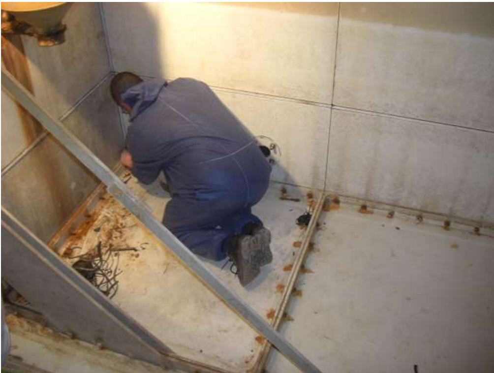
These pictures show the tank having been drained of all water and the COVAC Operative cutting back the now failing mastic used between the sectional GRP panels.
