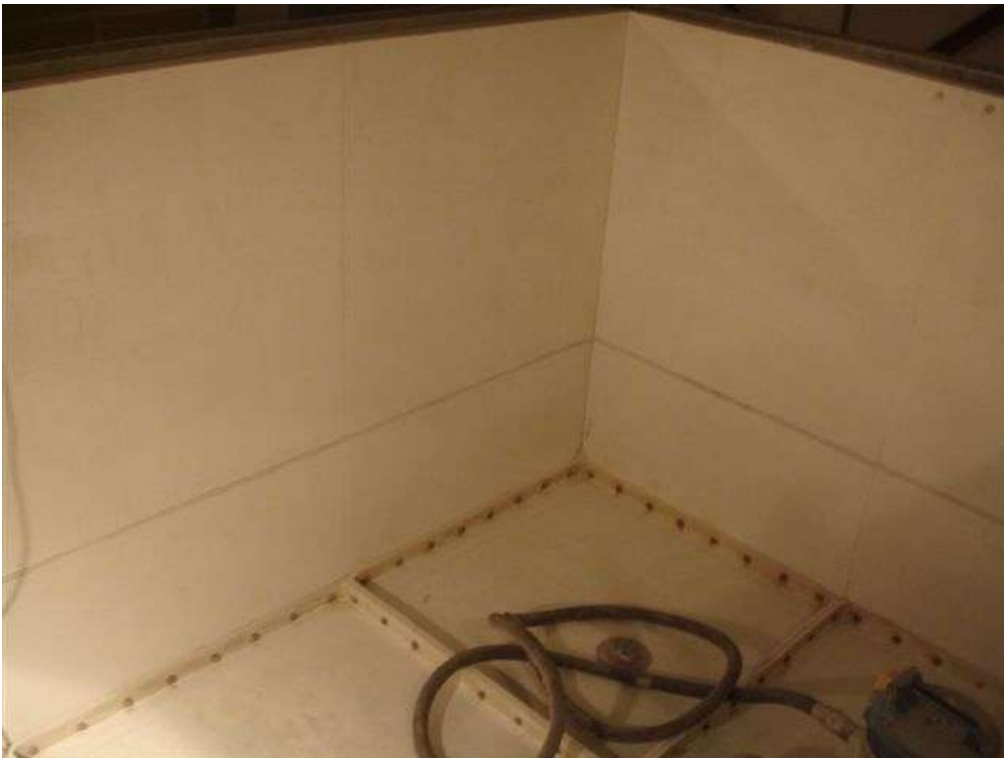
The pictures here show the internal substrate of tank # 1 both during and after preparation by the COVAC Operatives, to ensure that a suitable surface profile was raised for the 3M coating system to adhere to.
