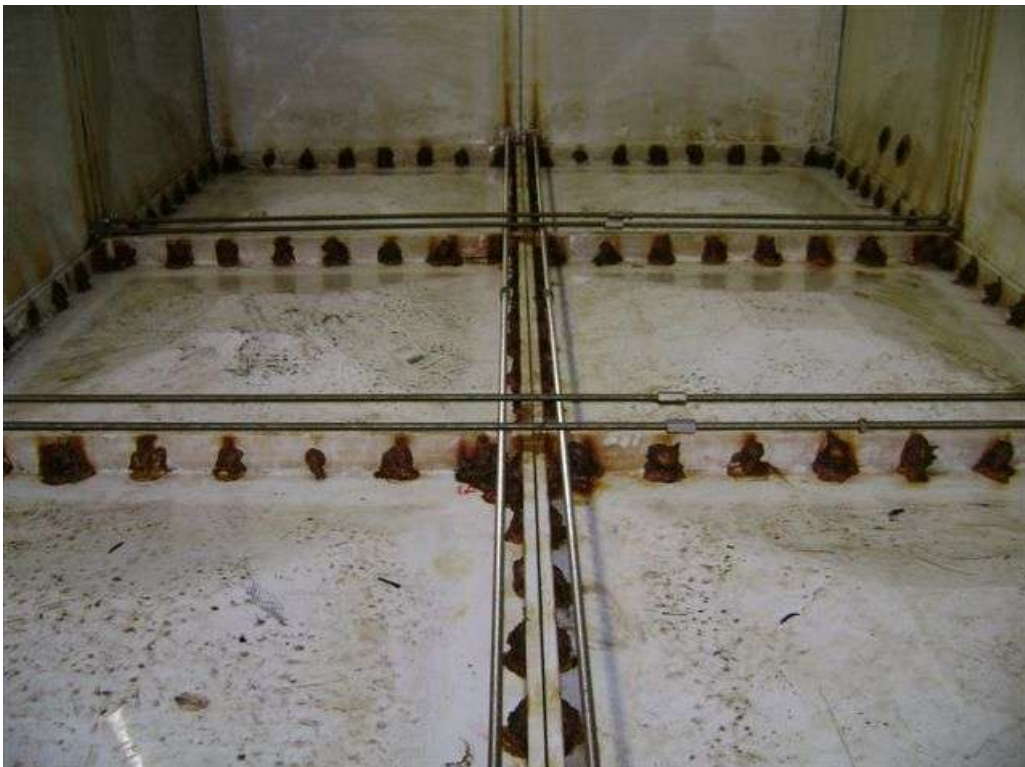
These photographs show the internal surfaces of the tank having been drained of water, but prior to any work commencing. Severe corrosion on the steel fastenings can be clearly seen.
