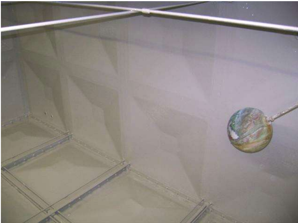
The following photographs show the final application of t 3M Scotchkote™ 165PW (grey).
