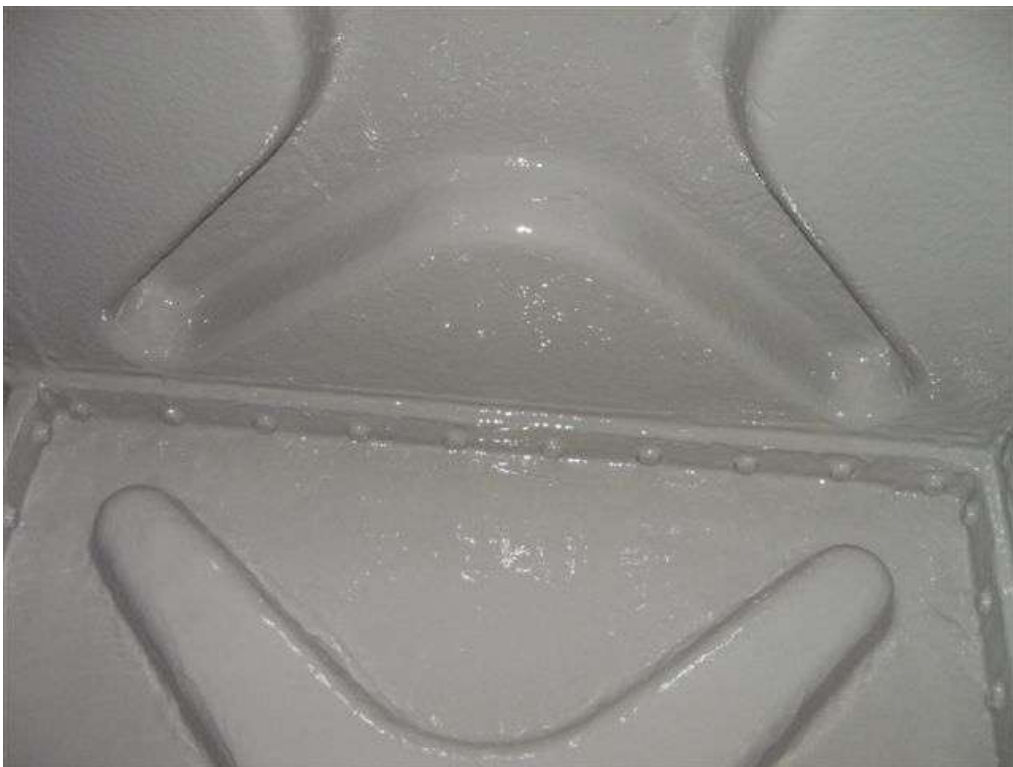
The following photographs show the final application of 3M Scotchkote™ 165PW (grey).
