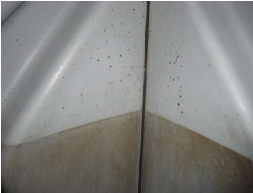
Black spore fungi can be clearly seen and there is also evidence of small blisters developing in the gel coat.
