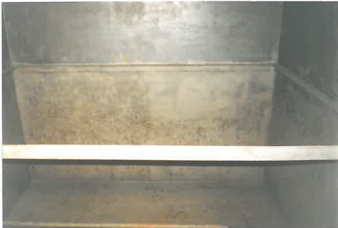
Both tanks were internally dry grit blast cleaned to a minimum SA 2.5 BS7079 Part A1 1989 i.e. complete removal of all existing coating and corrosion.
