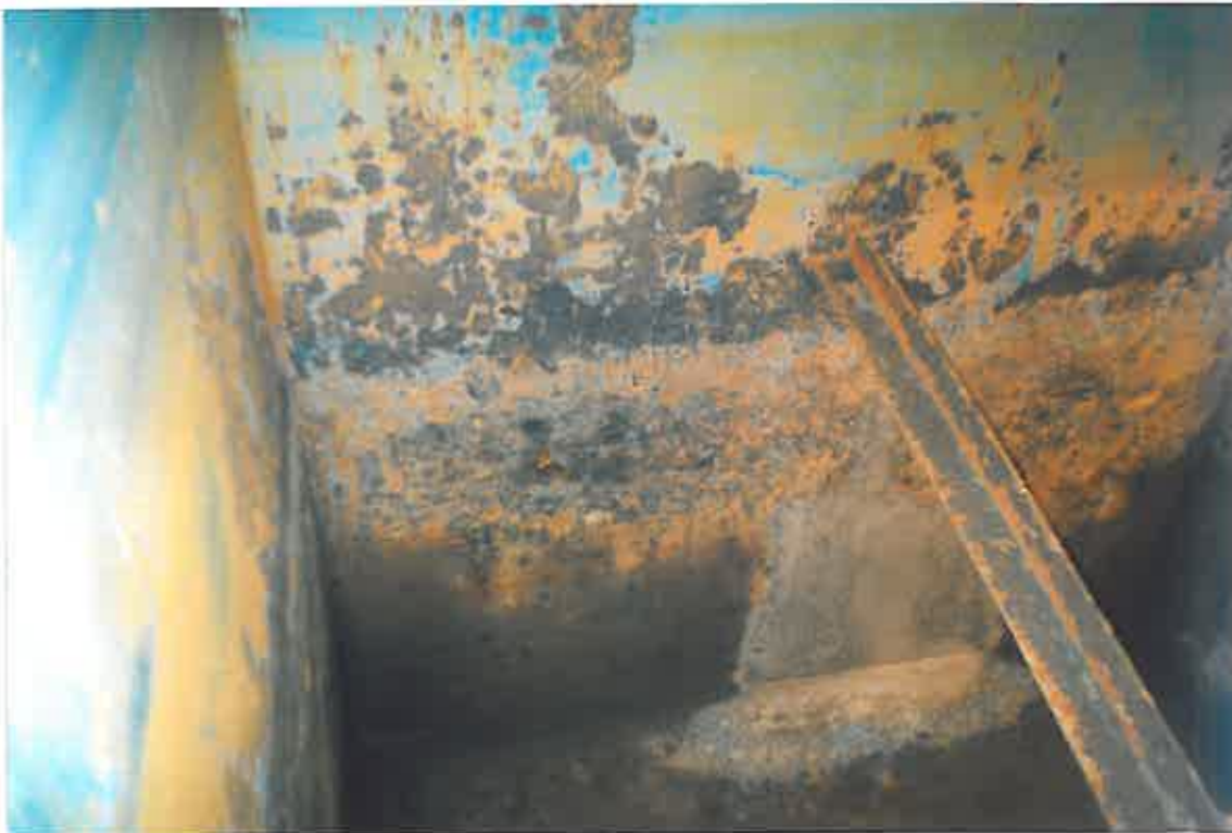
The main boiler house, hotwell tank and towers ring hotwell tank were previously internally coated with a blue epoxy coating which had now come to the end of its useful life.
