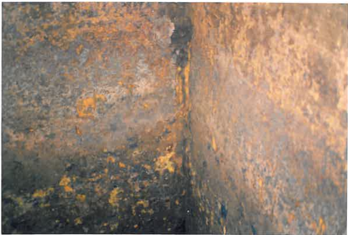
The above and following photographs show the internal condition of the tank prior to refurbishment.
