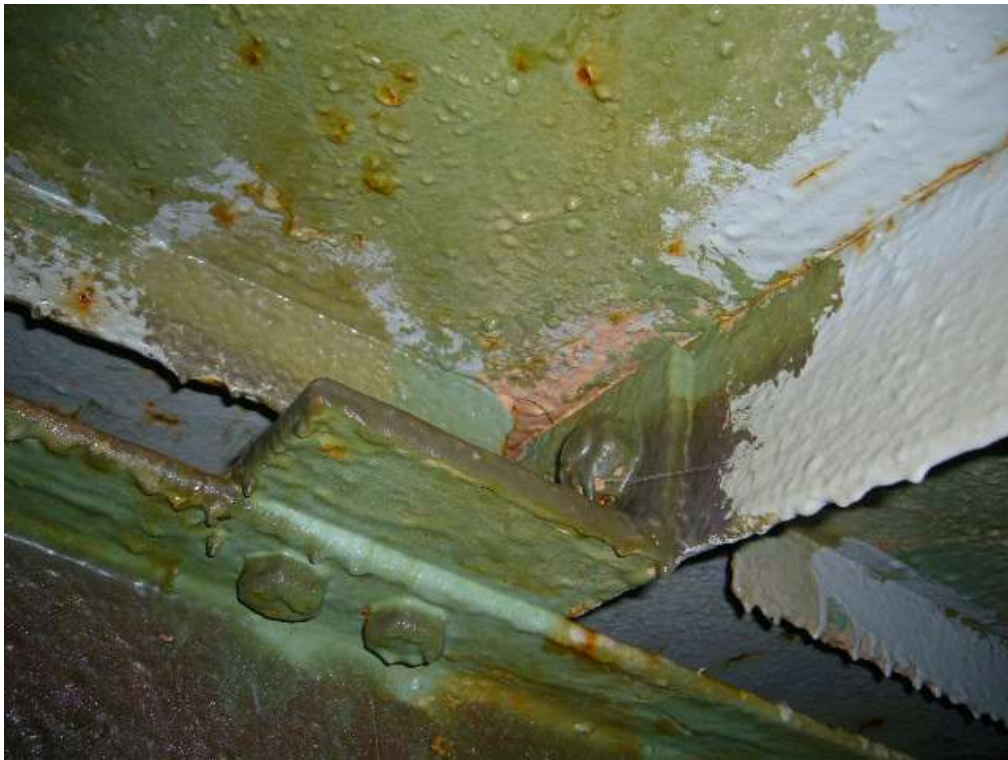
These photographs show the internal surfaces of structure having been drained of water and prior to any preparation works being carried out.
