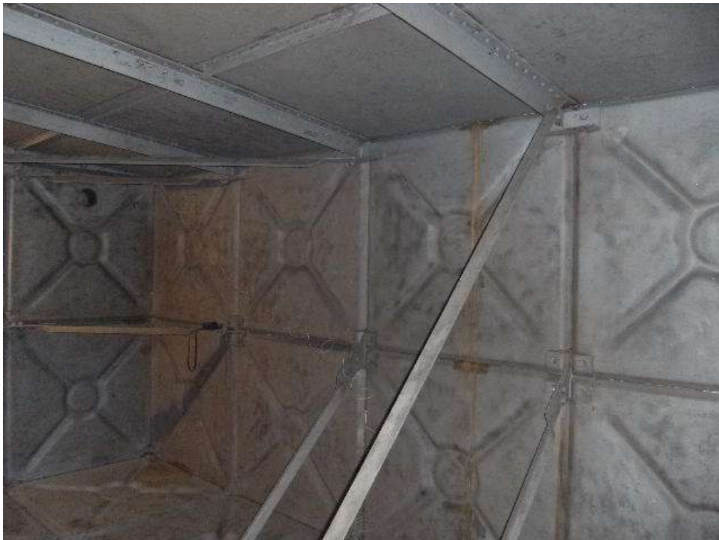
These photographs show the internal surfaces, after the mechanical preparation process by the COVAC Operatives using dry abrasive grit blast equipment in accordance with the a accepted Standard.
