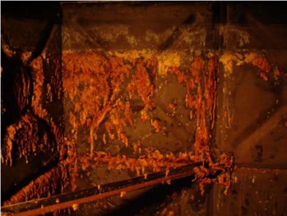
These images show internal condition of tanks having been drains, but prior to any refurbishment work commencing.
