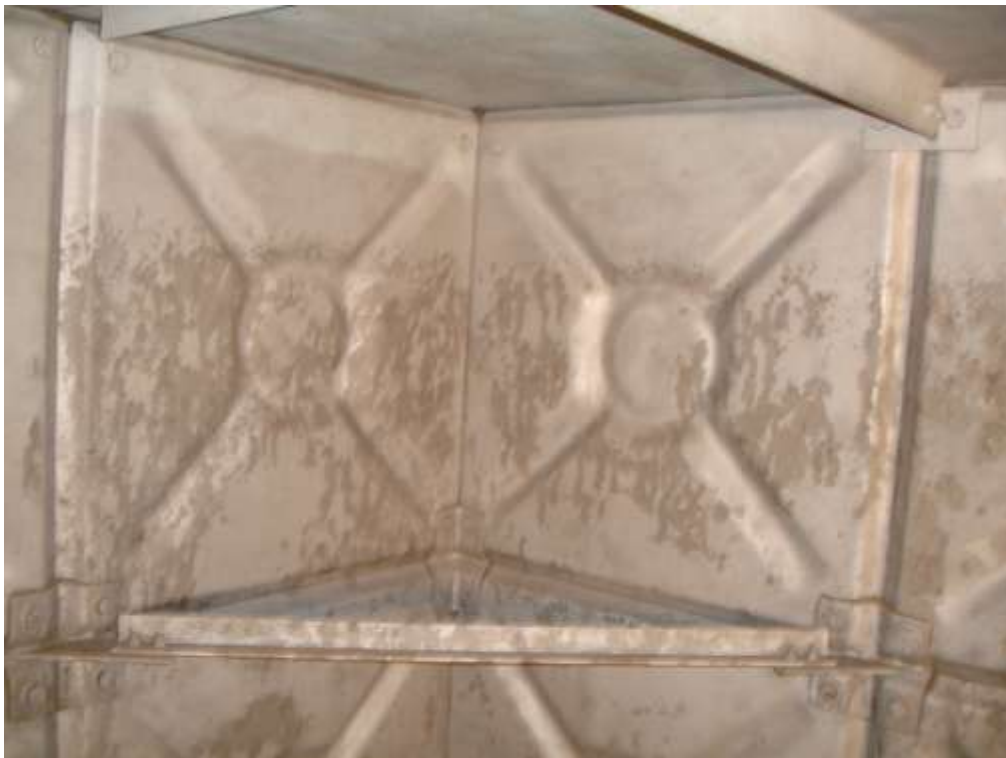
These photographs show the internal surfaces of the tanks after mechanical preparation by the COVAC Operatives, using dry abrasive grit blast equipment in accordance with the accepted Standard.
