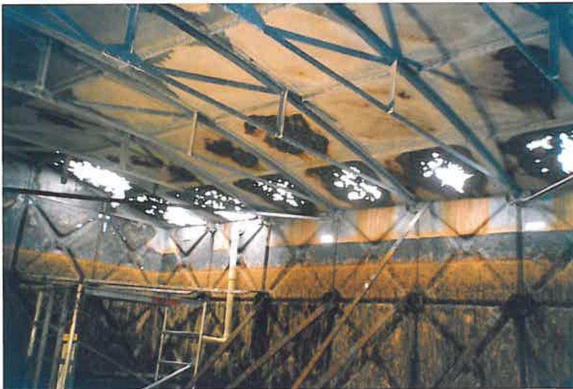
These photographs show how the corrosion had attacked the steel roof. These holes were eventually cut to firm edge, prior to being repaired utilizing new flat, steel, galvanised sheeting.
