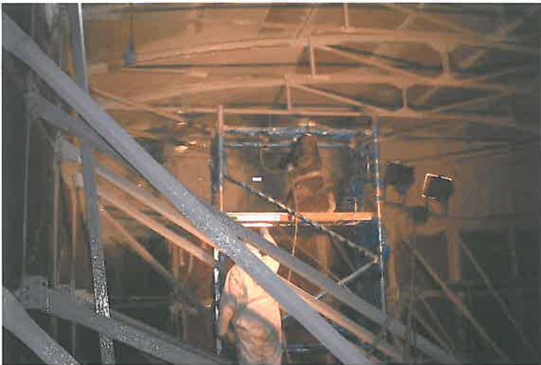
These photographs show COPON Hycote 165 PW Solvent Free Polyurethane being spray applied by means of Plural Component, Hot Applied Spraying Equipment.
