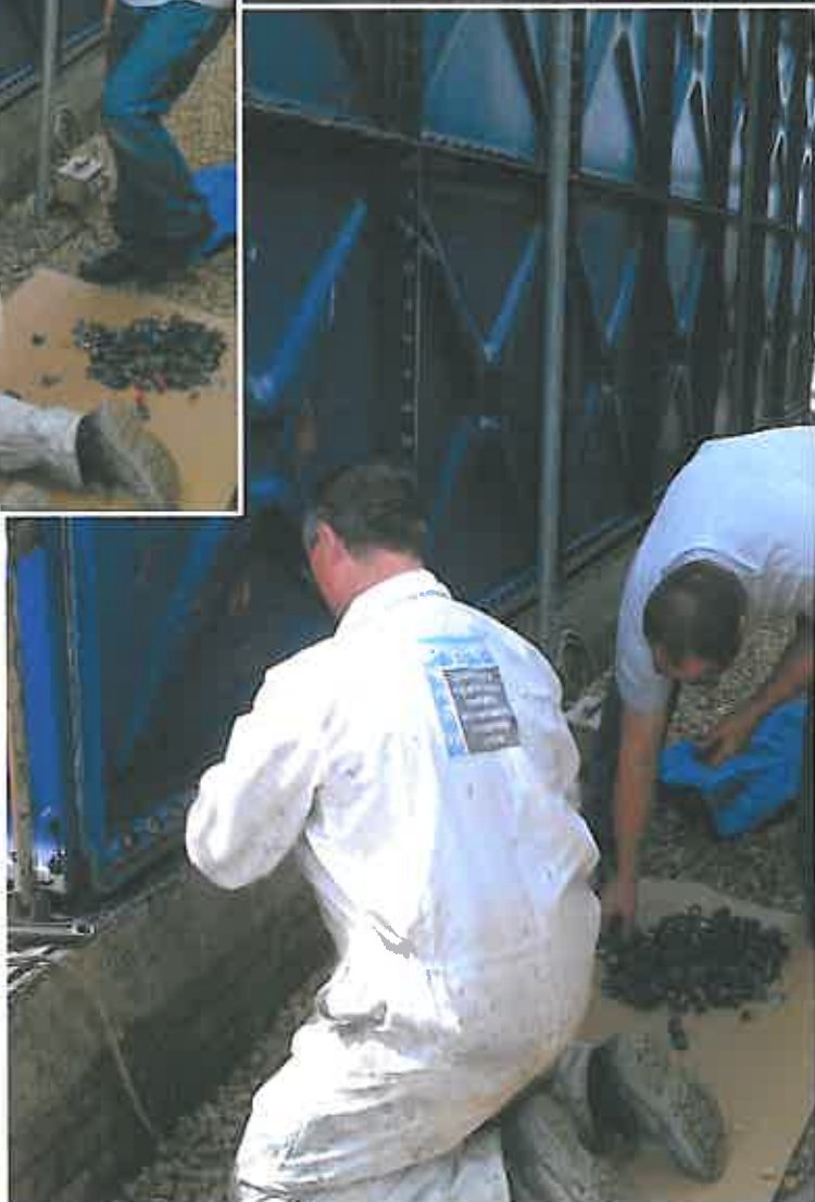
These photographs show the bottom panel (having been prepared and re-lined) being replaced by our operatives.
