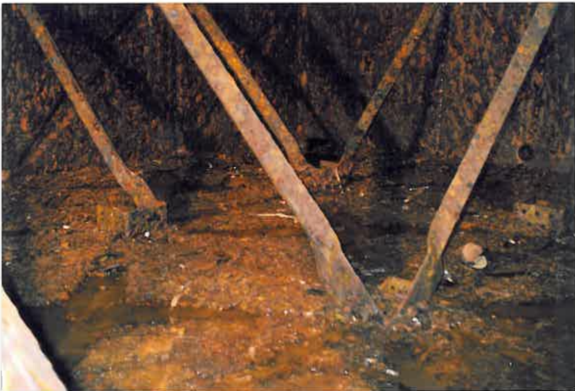
These photographs show the severity of the corrosion to the internal surfaces of the tank.
