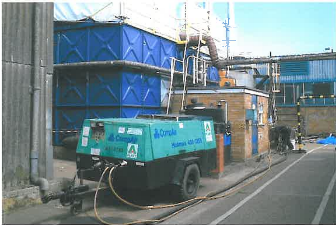
These photographs show the Plural Component, Spraying Equipment, located near to the access point of the tank.
