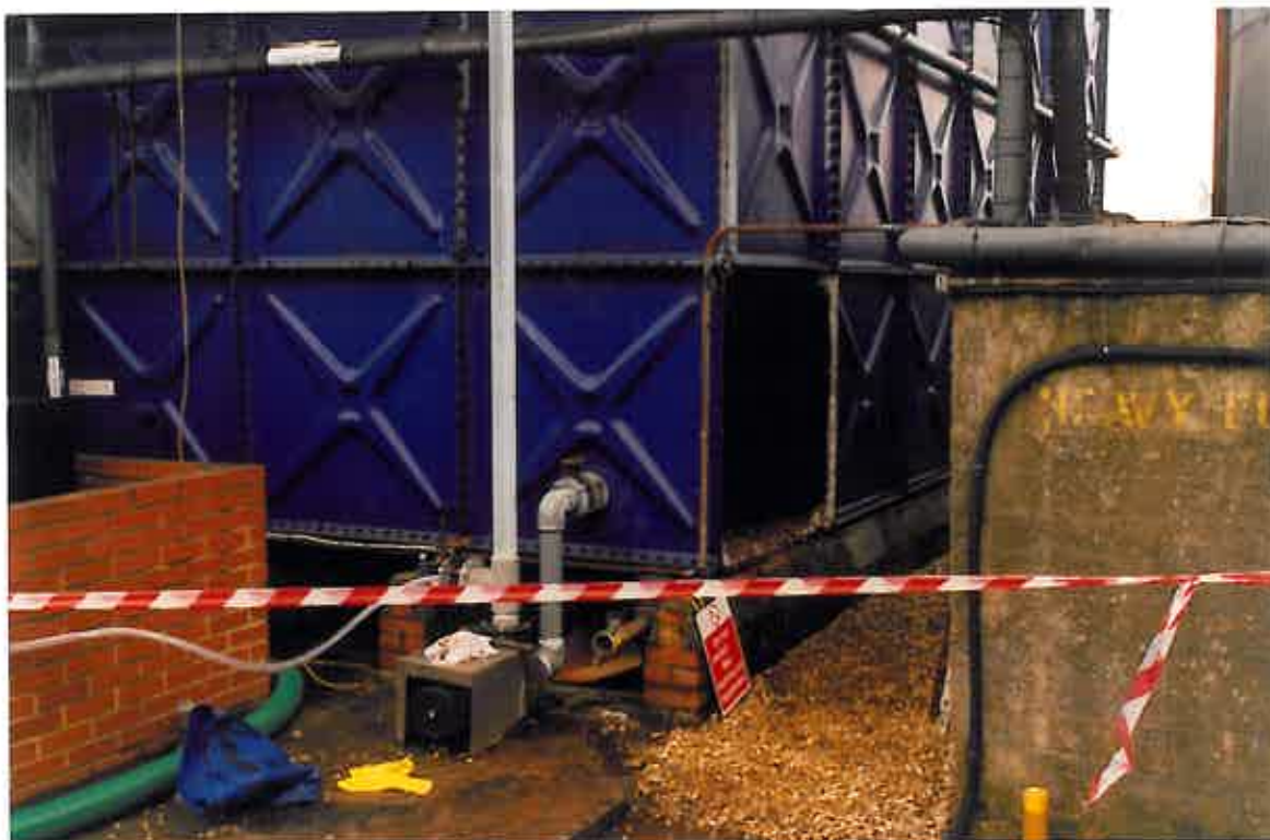
These photographs show the removal of one of the bottom, sectional panels from the tank. This was a vast improvement on the original roof entrance point in terms of ease of access and health and safety aspects.
