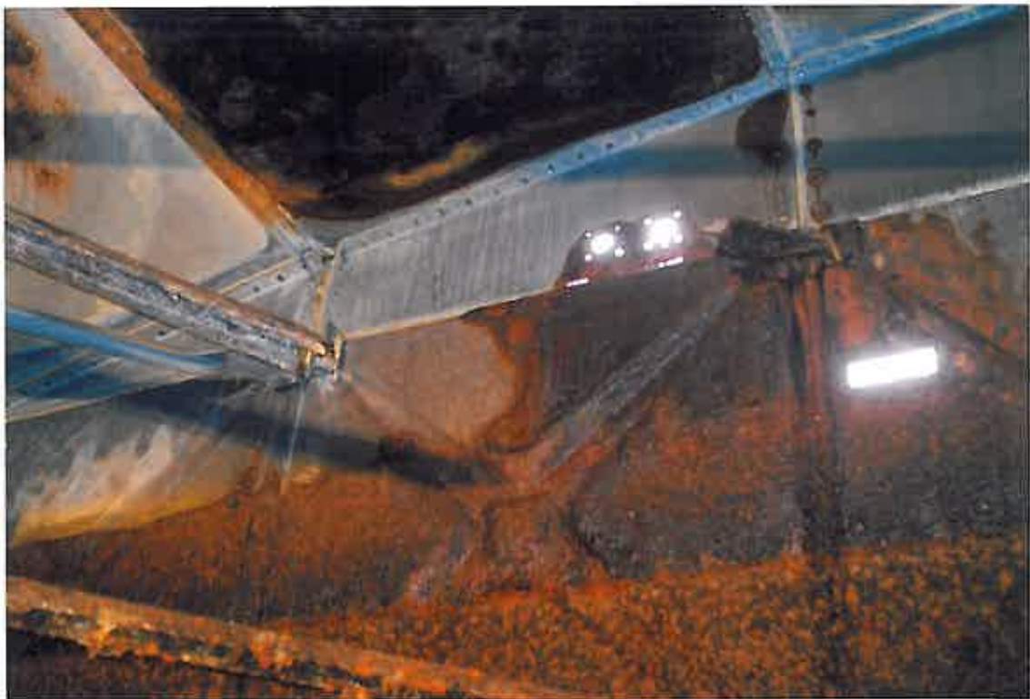
These photographs show the extent of damage caused to at least eight of the steel, support struts of the tank. These struts were made good by welding approximately sized angle iron to damaged areas.
