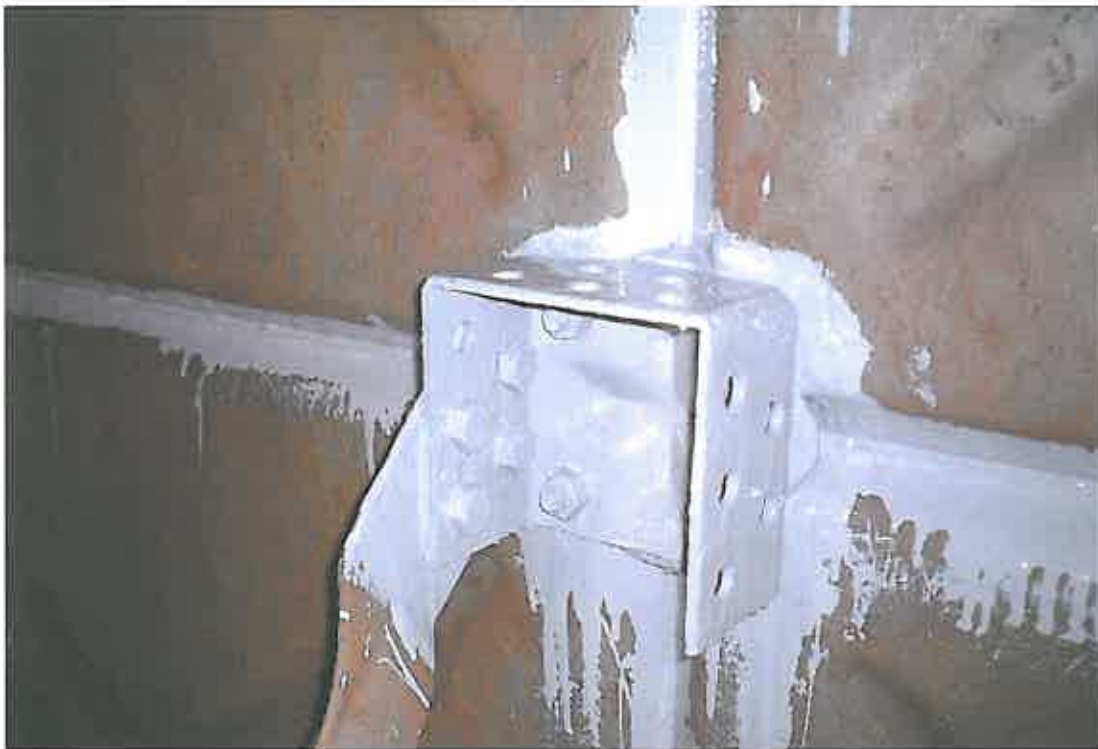
These photographs show the 'stripe coating' (by means of brush) of all welds, joints, edges, bolt heads and other sharp protuberances in order to maintain the specified film thickness to these areas.
