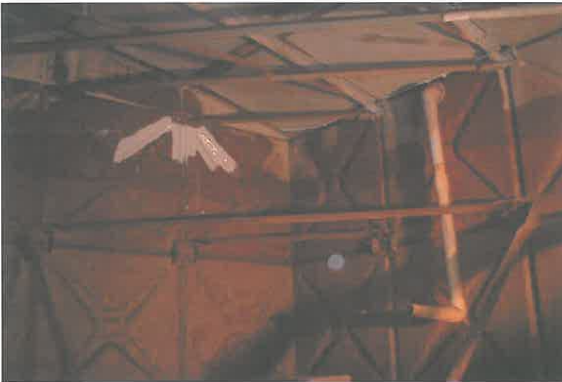
These photographs show the larger holes above the oxygen exchange line being repaired, utilizing a combination of COPON Hycote 165 PW and fibreglass webbing.
