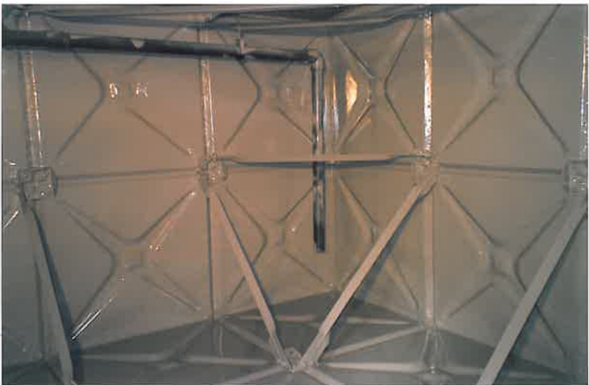
These photographs show the internal substrate of the tank, having been completely lined with COPON Hycote 165PW Solvent Free Polyurethane to a nominal w/dft of 1000 microns (1mm) by means of Plural Component, Hot Applied, Spraying Equipment.
