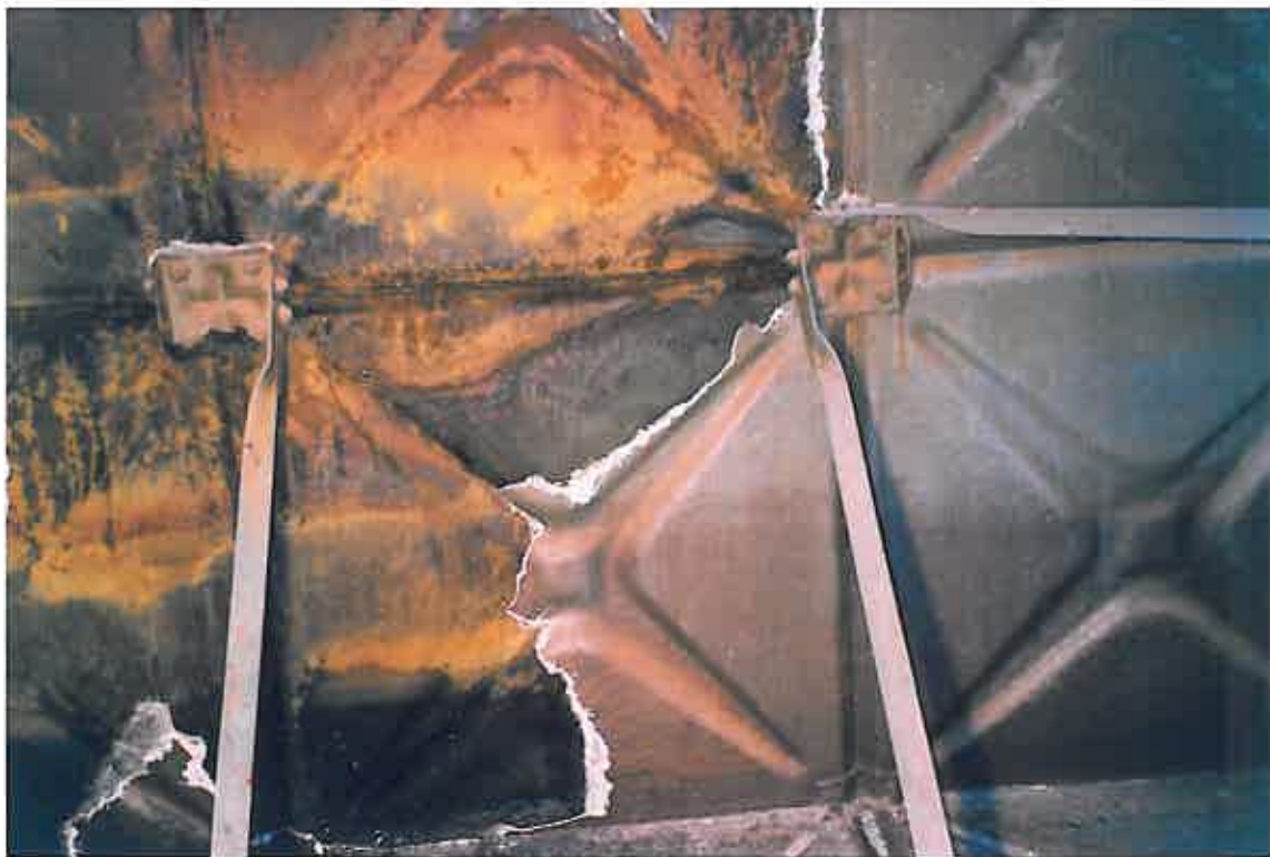
These photographs show our operatives in the process of removing the failed fibreglass lining system utilizing tools such as pneumatic chisels. This process of removal revealed a Bitumen paint underneath.
