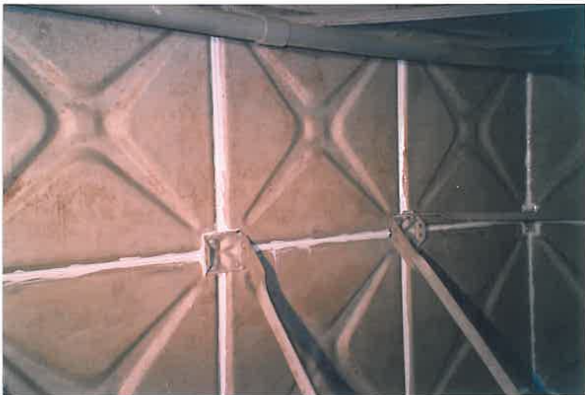
These photographs show the initial stripe coating, by brush application, of all areas such as joints, sharp edges, struts, bolt heads, ladder, etc.
