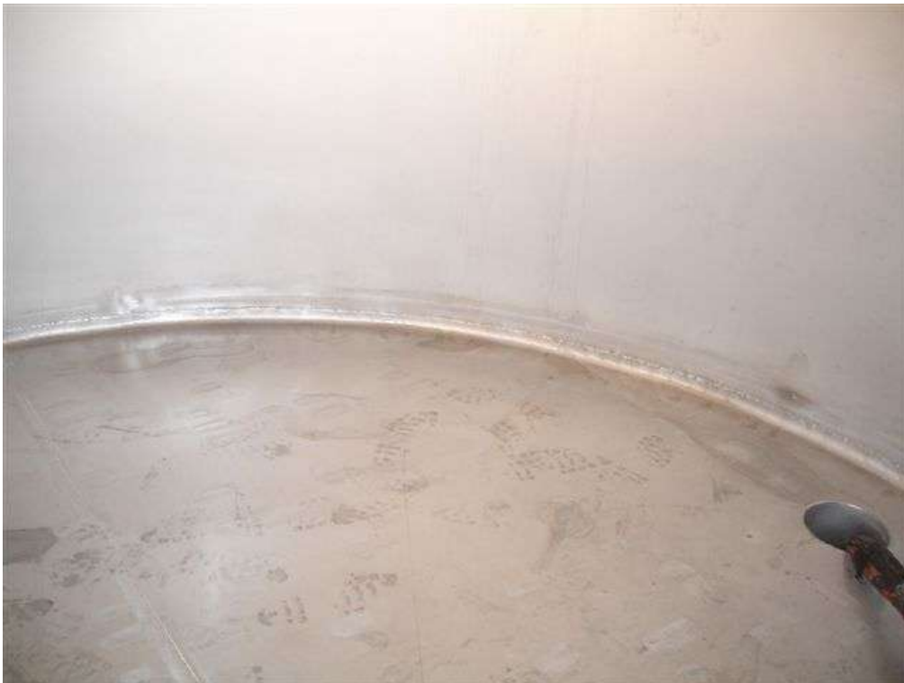
These photographs show the internal surfaces of the tanks prior to any work commencing.
