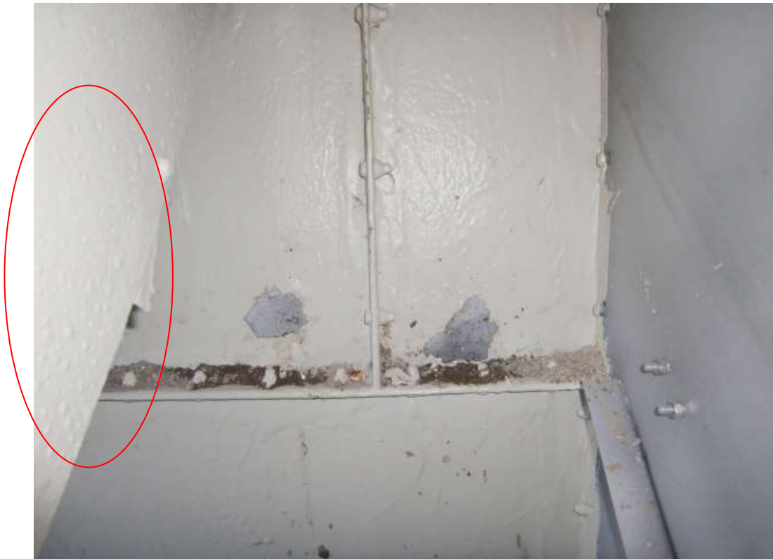
These photographs show the internal substrate of the tower prior to the relining work commencing. Blistering of the existing coating can be clearly seen.
