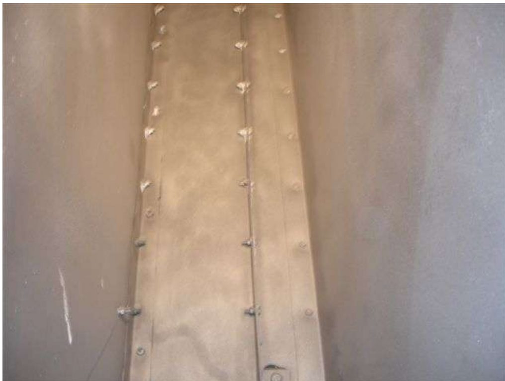
The pictures show the internal substrate after being prepared by COVAC Operatives using dry abrasive blasting equipment.
