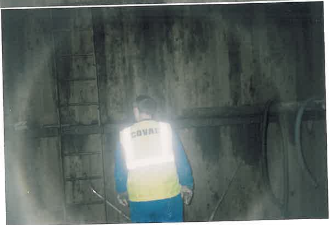
These photographs show the internals of the tank having been drained of water and prior to any preparation works.
