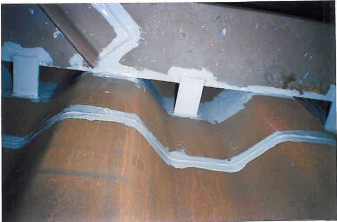
These photographs show all weld joints, sharp edges, struts, etc having been 'stripe coated' by brush.
