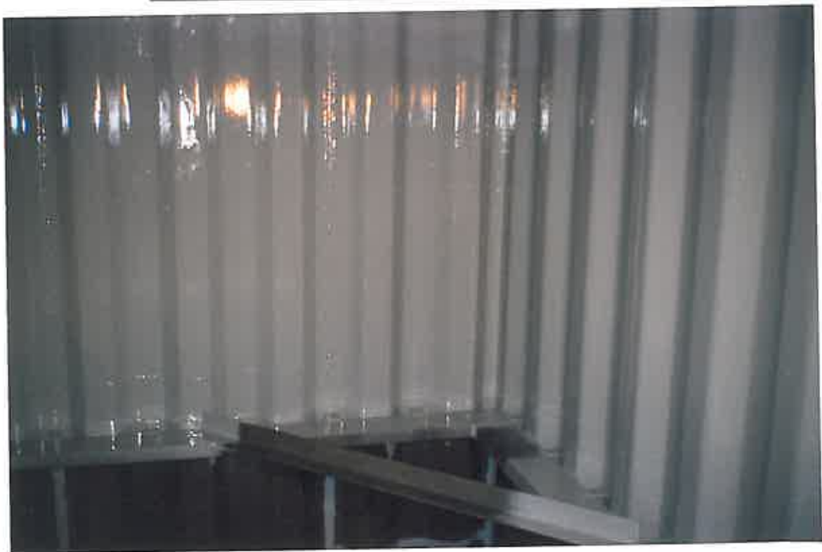
These photographs show the 'stripe coating' being overcoated with one full coat of 165 PW being applied through twin component, hot applied specialist spray equipment.
