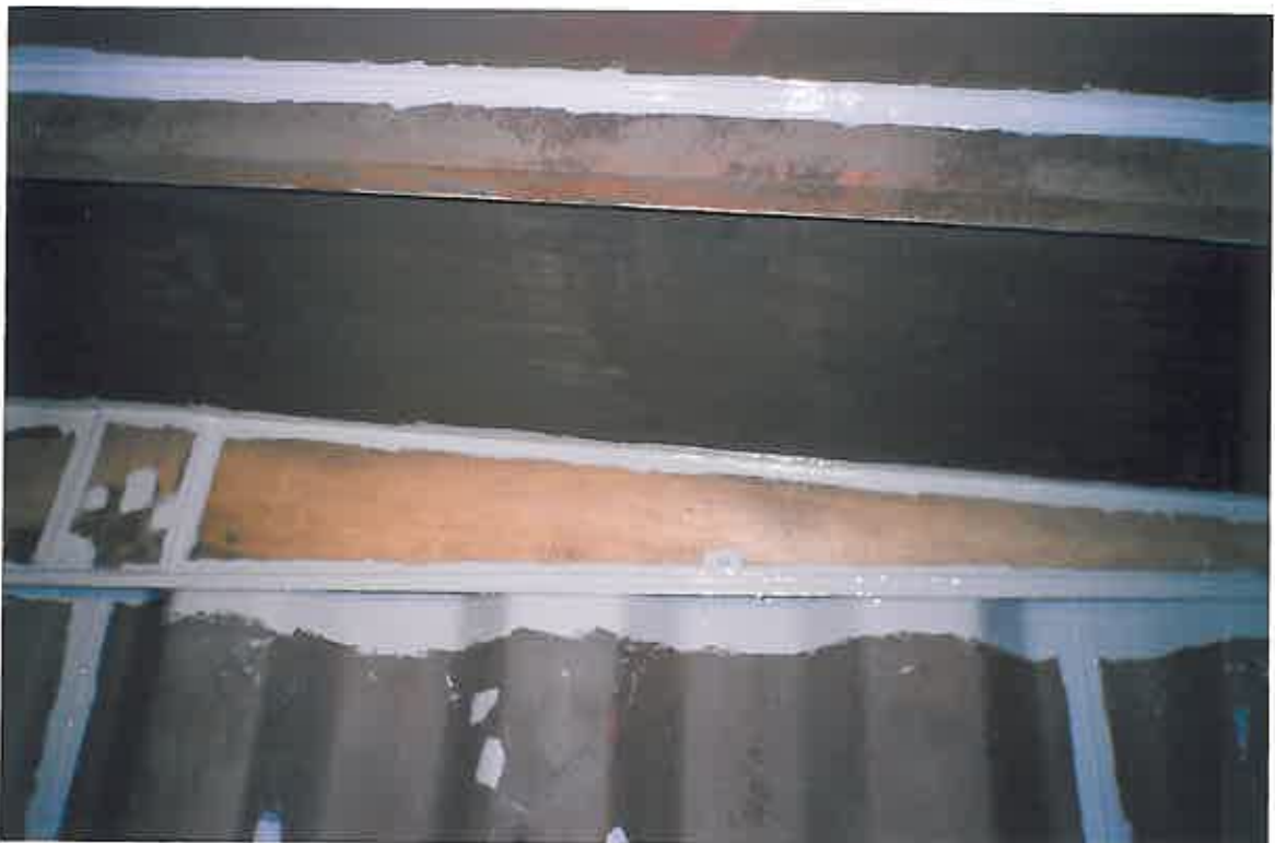
The above photograph also shows the wooden boarding required in order to prevent cross contamination of the two tank compartments whilst the preparation and re-lining was taking place.
