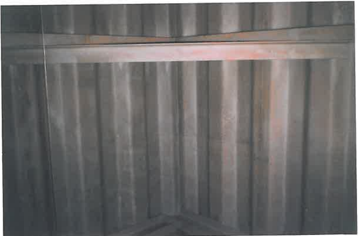
These photographs show the internal surfaces of the tank having been prepared by means of dry abrasive blasting technique.
