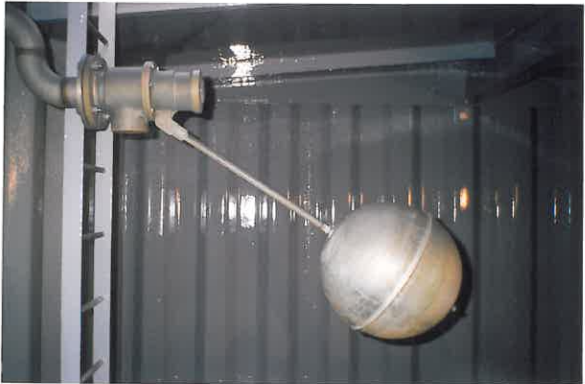
These photographs show the internal surfaces of the tank having been completely re-lined with COPON Hycote 165 PW Solvent Free Polyurethane utilizing, twin component, hot applied, specialist spray equipment.
