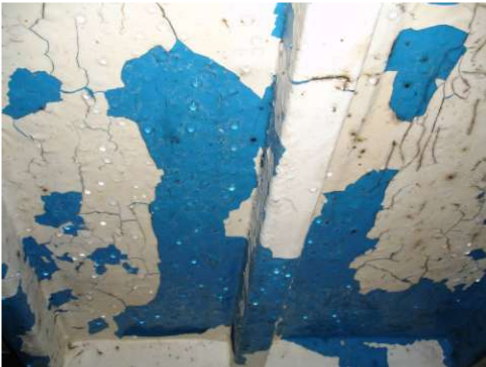
These photographs show the internals of the tanks, prior to any preparation work. The photographs clearly show the deterioration of the epoxy coating and delaminating of the GRP lining.
