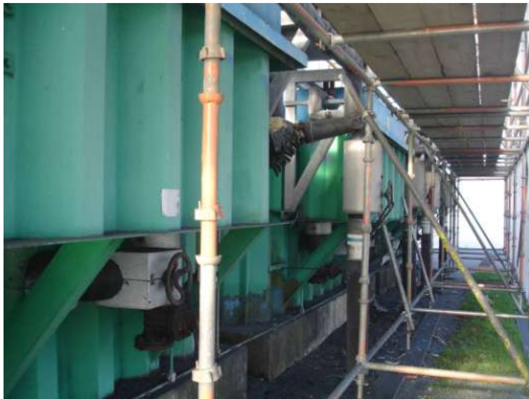
These images show the external of the tanks prior to any preparation work by our site operatives.
