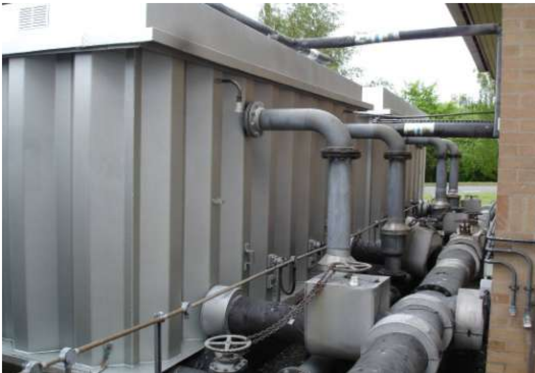
The areas not required to be coated were initially masked off prior to the 2no. coats of airless spray application. The following photographs show the completed coated external surfaces of the tanks of metallic silver coloured COPON Hycote 152LV to a Dry Film Thickness of 500 Microns.
