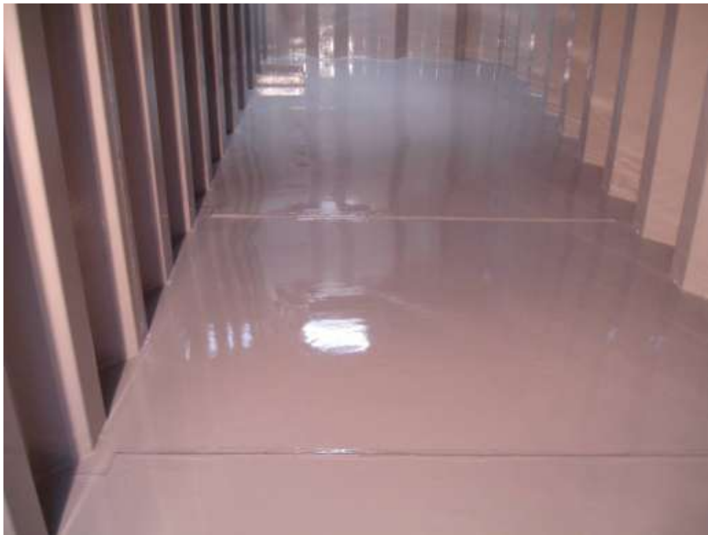
The following photographs show the tank steel substrate having been fully coated with COPON Hycote 165PW Solvent Free Polyurethane (cream).
