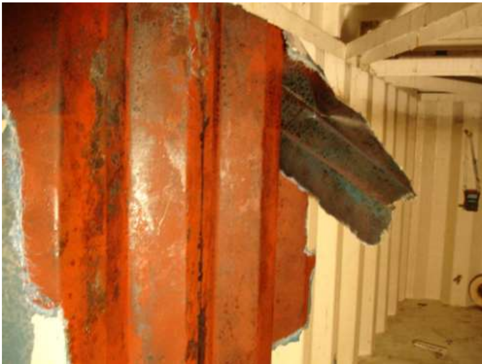
The following photographs show the GRP lining, which had to be removed utilising mechanical chisels revealing the epoxy coated steel substrate.
