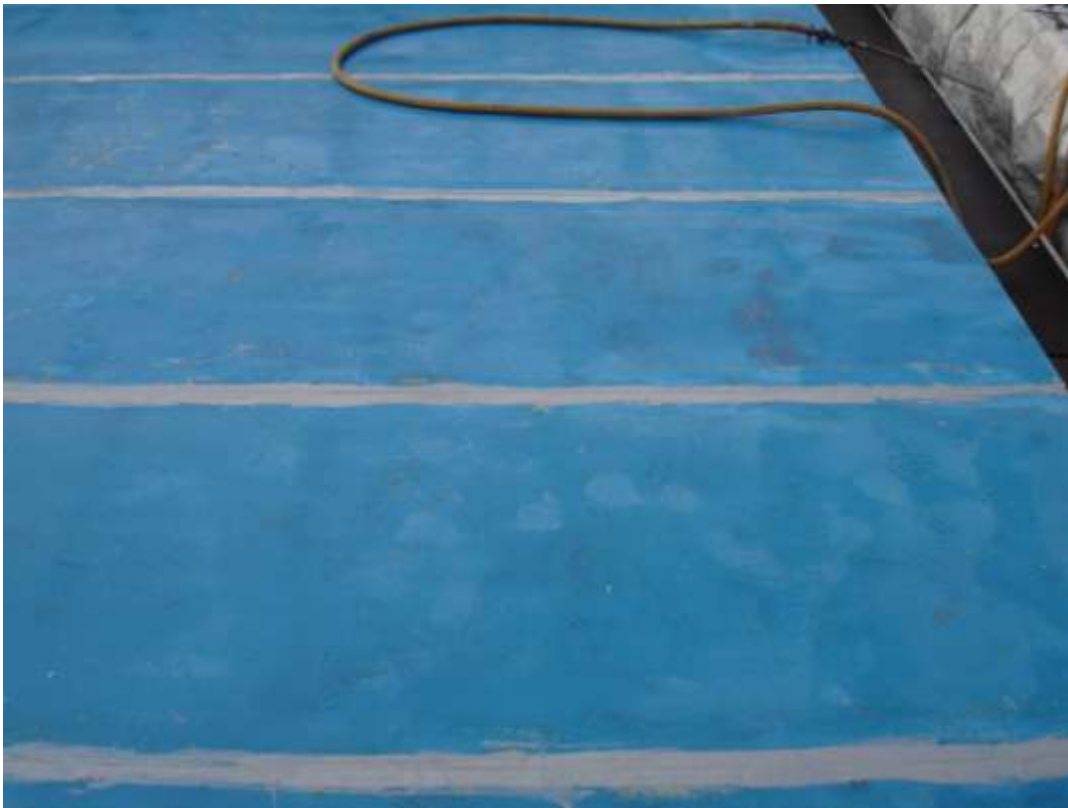
These images show the GRP roof having been resealed and stripe coated prior to the manual application of COPON Hycote 152LV.
