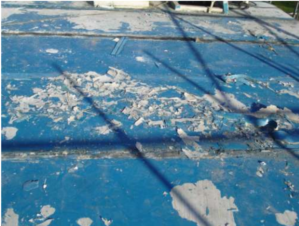
Originally, the GRP lid was coated in an epoxy paint, which had begun to delaminate and the above photographs show the roof preparation work in the manual removal of the failed coating.
