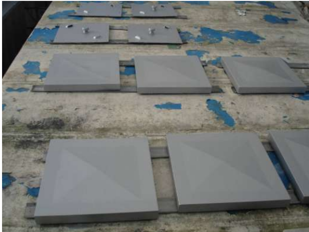
The following photographs show the roof being manually coated with COPON Hycote 152LV High Performance Coating.
