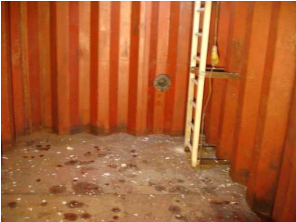
These images are of the internals of the tanks after the GRP lining has been removed from all internal surfaces.
