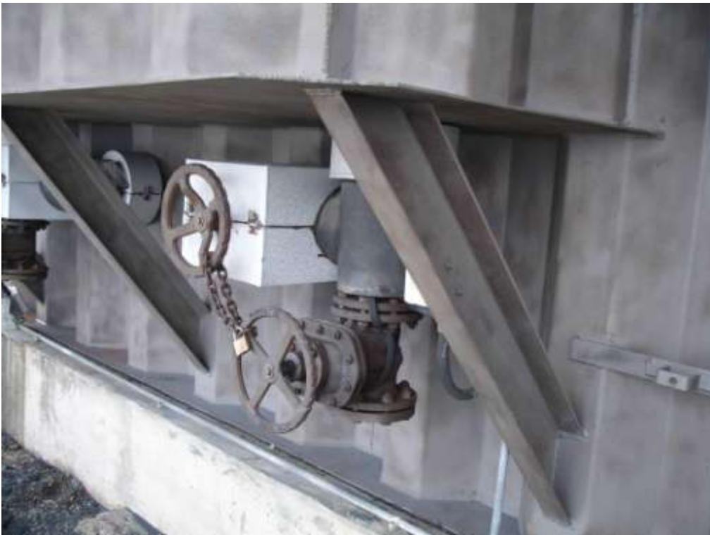
The following images show the exterior steel surfaces after having been prepared by COVAC operatives by means of dry abrasive grit blasting equipment in order to achieve the required surface profile for adherence of the COPON Hycote 152LV Coating System.
