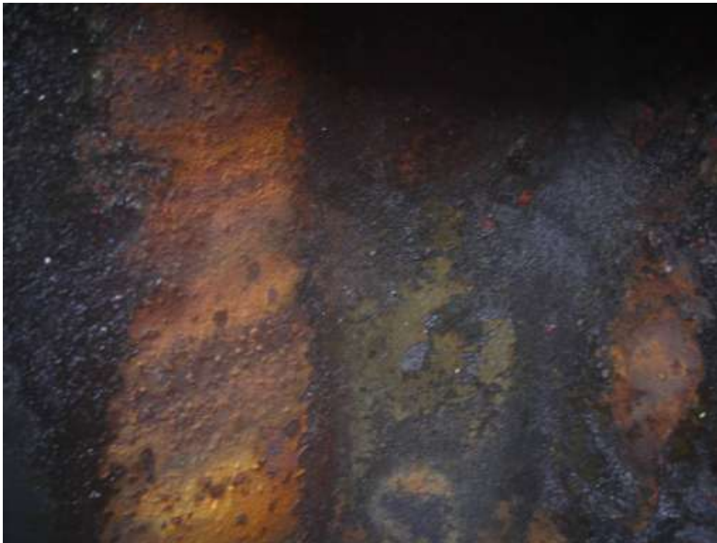
The photographs above clearly show progressive corrosion to the steel due to moisture entrapment between the steel and GRP lining substrates.
