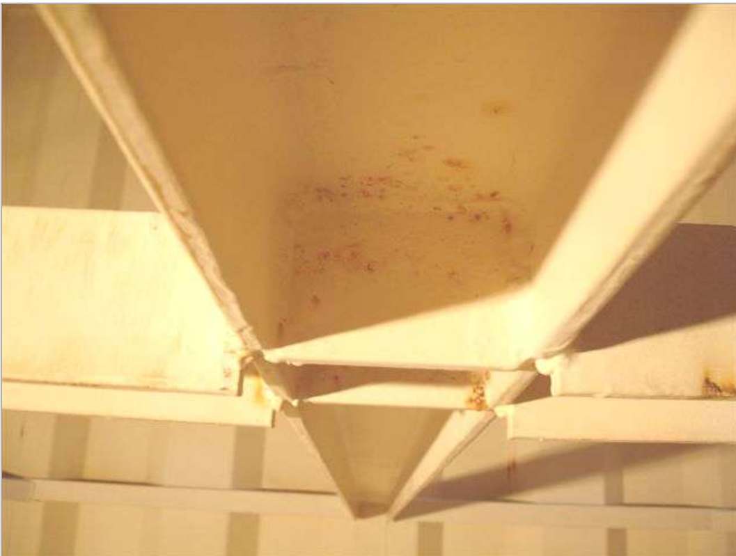
These photographs show the internal substrate of the compartment having been drained of water, but prior to the relining work commencing.
